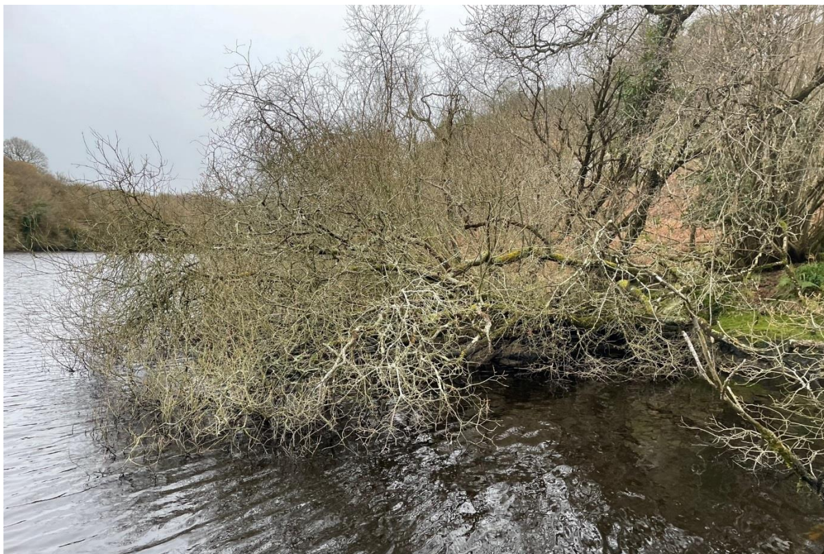
Over-hanging trees in narrow river section at Poulaphuca Station
