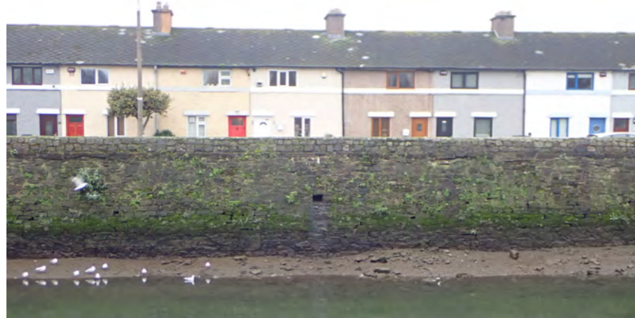
East Wall Road Sea Wall opposite Fairview Park Source: ADCO for DPC
