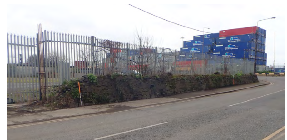
Parapet of the GSW stands today as a low boundary wall on Pigeon House Road in close proximity to the operational port, and has been breached in many places Source: ADCO for DPC
