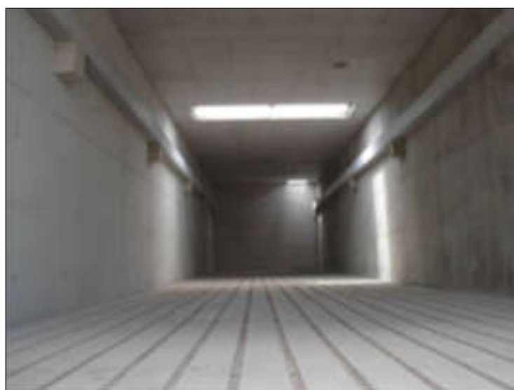
Figure 4-7: Typical composting tunnel with spigot floor
