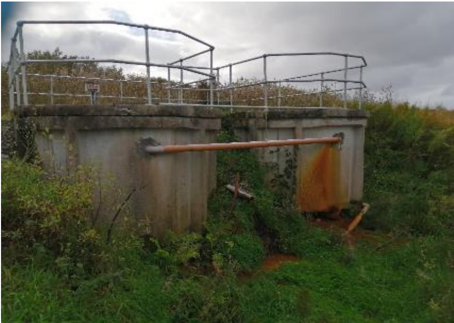
Picture 10 Leachate Collection Tanks
