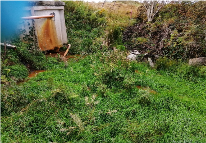
Picture 7 Overflow pipe from the leachate storage /pumping tanks
