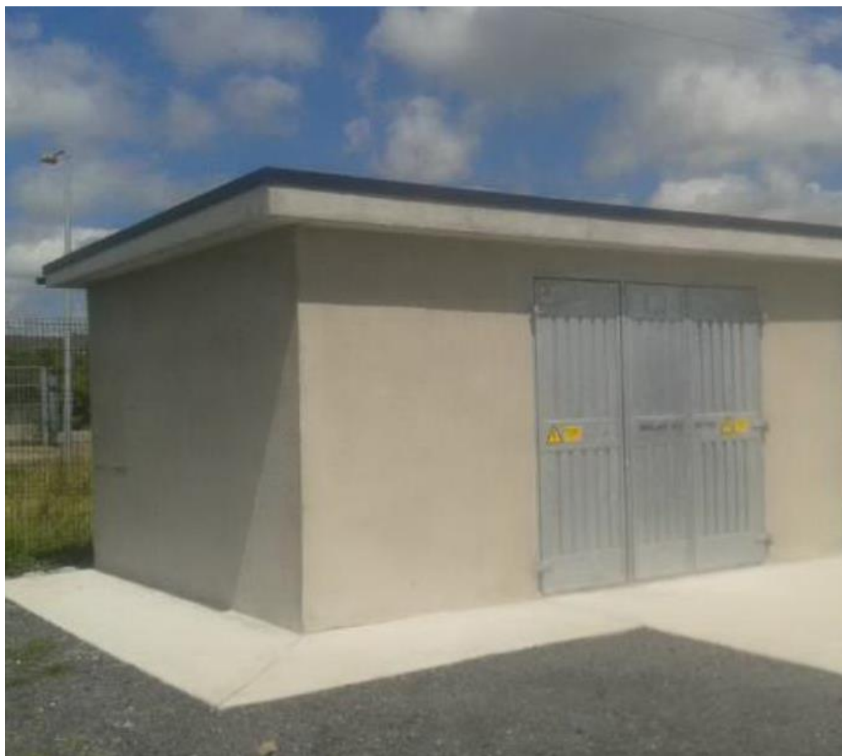
Plate No 1: Example of single mv electrical substation
