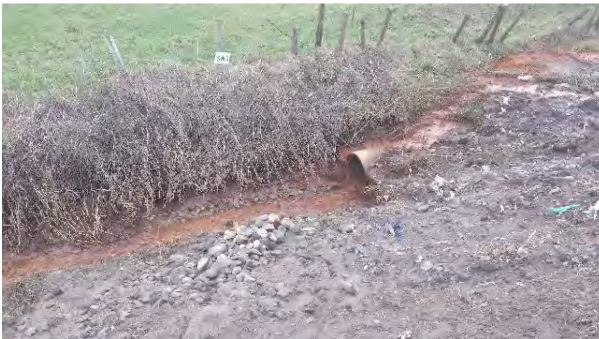
Figure 8.9 Leachate Impact within Northeastern Boundary Drain pre-restoration
