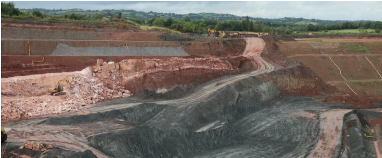
Figure 4.2: Good surface runoff management practices at the Knocknacran open cast, including plating of the bench faces and drainage of the benches
