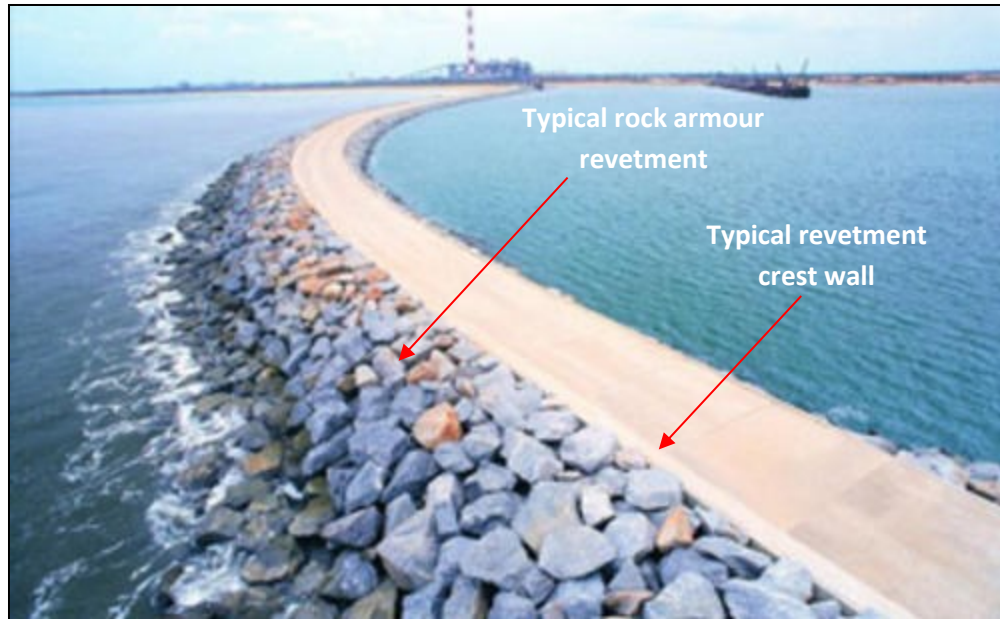
Figure 12 Example breakwater showing rock armour revetment and crest wall. Similar in construction to the proposed perimeter embankment.
