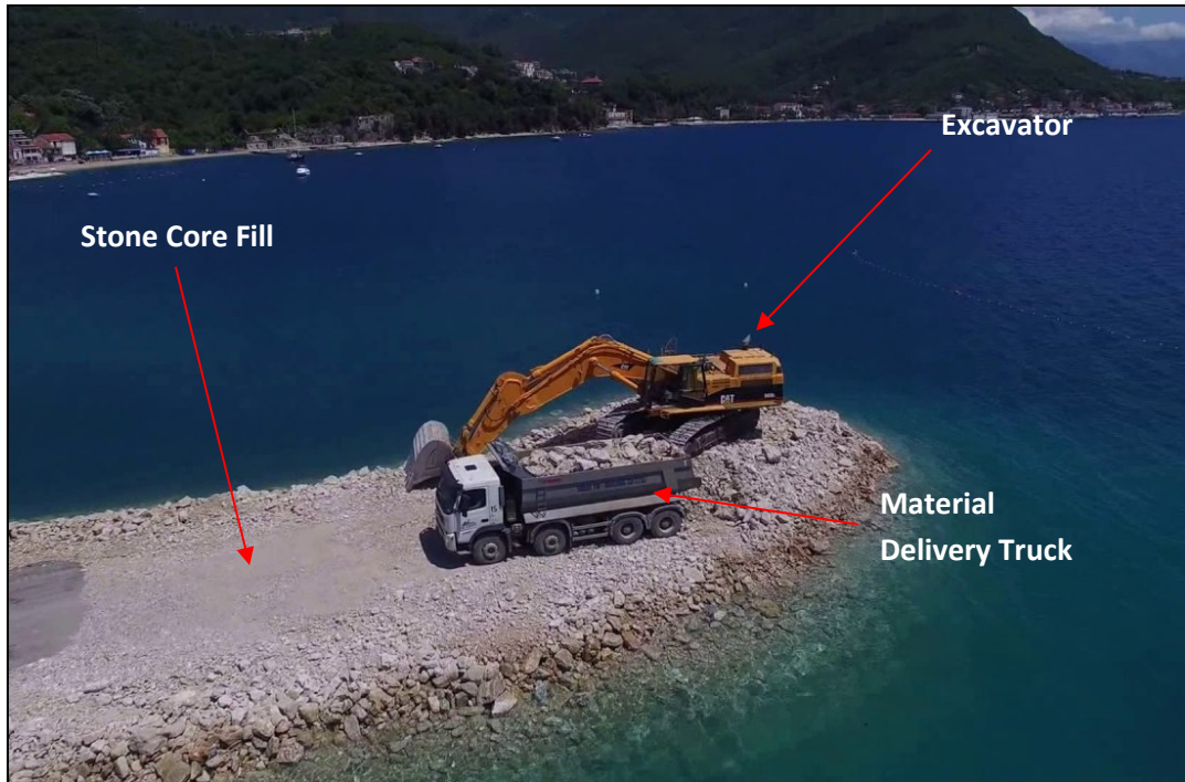
Figure 10 Shows typical operations for construction and embankment from land out into water.
