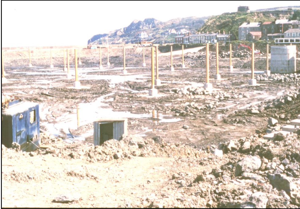
Figure 4 Construction of the marina area in the 1980s. Dredging was carried out in the dry.
