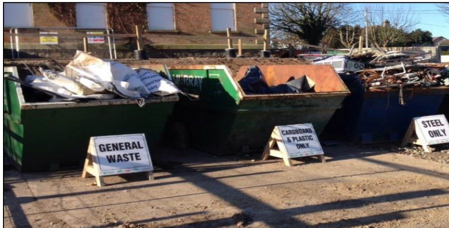
Figure 18 Example waste segregation arrangement
