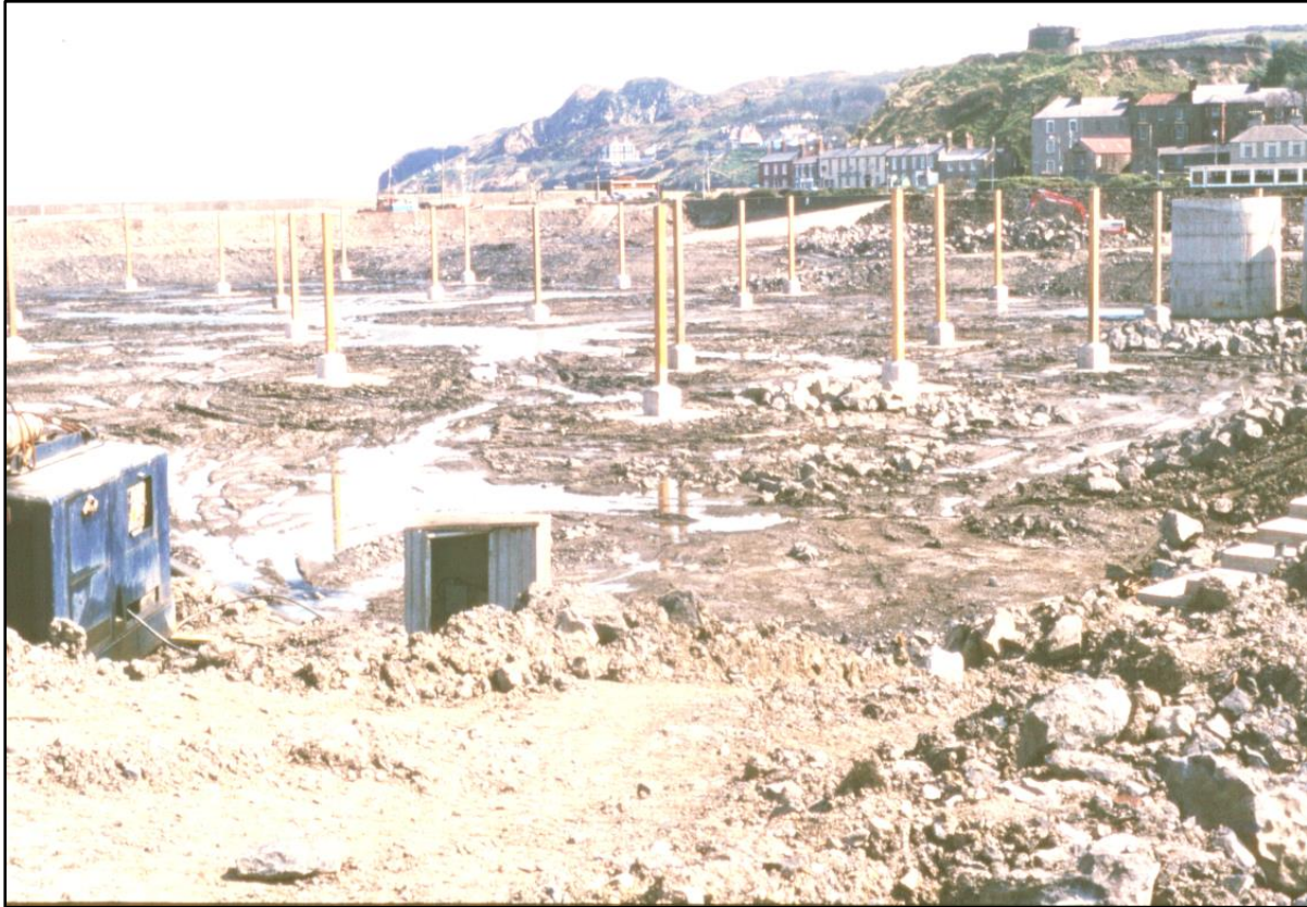
Figure 6 Construction of the marina area in the 1980s. Dredging was carried out in the dry.
