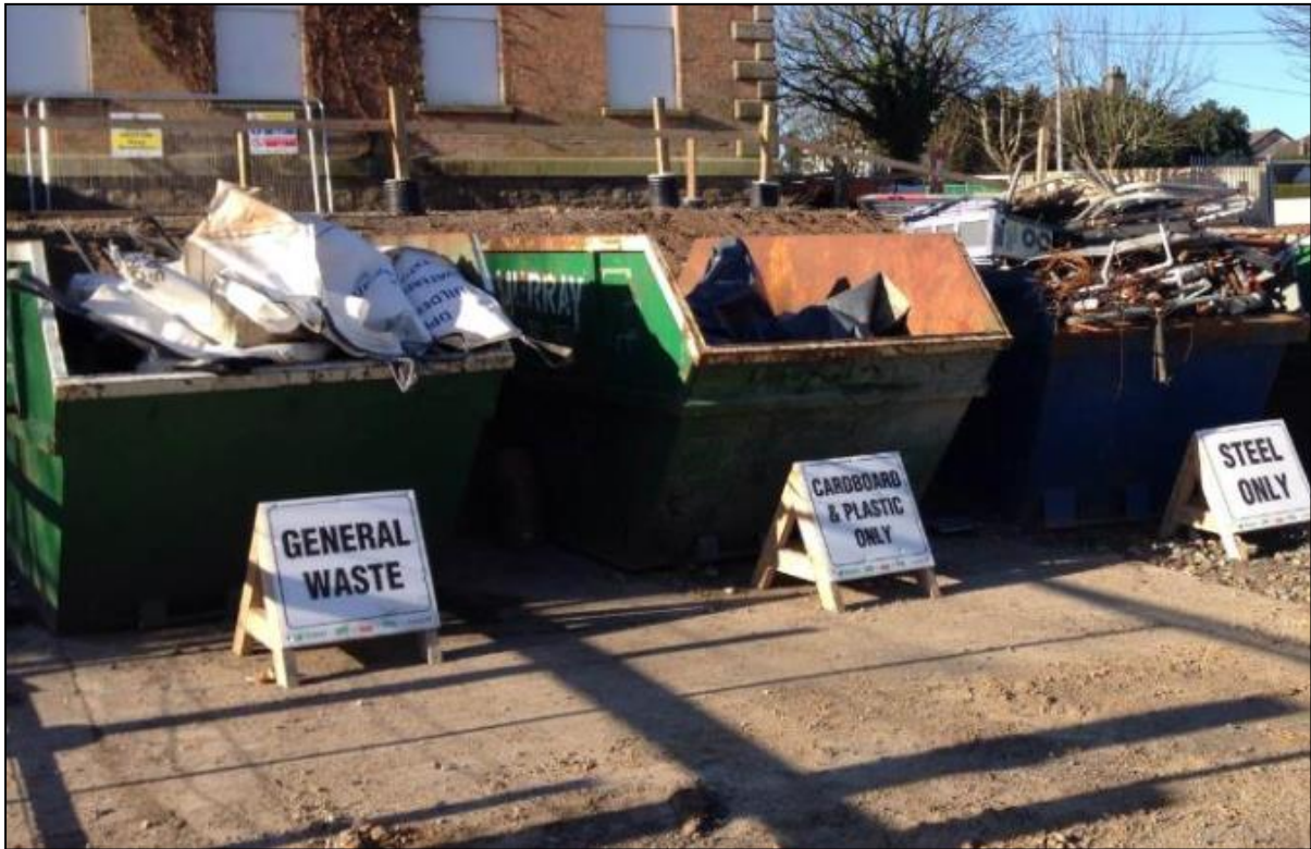
Figure 4 Example waste segregation arrangement
