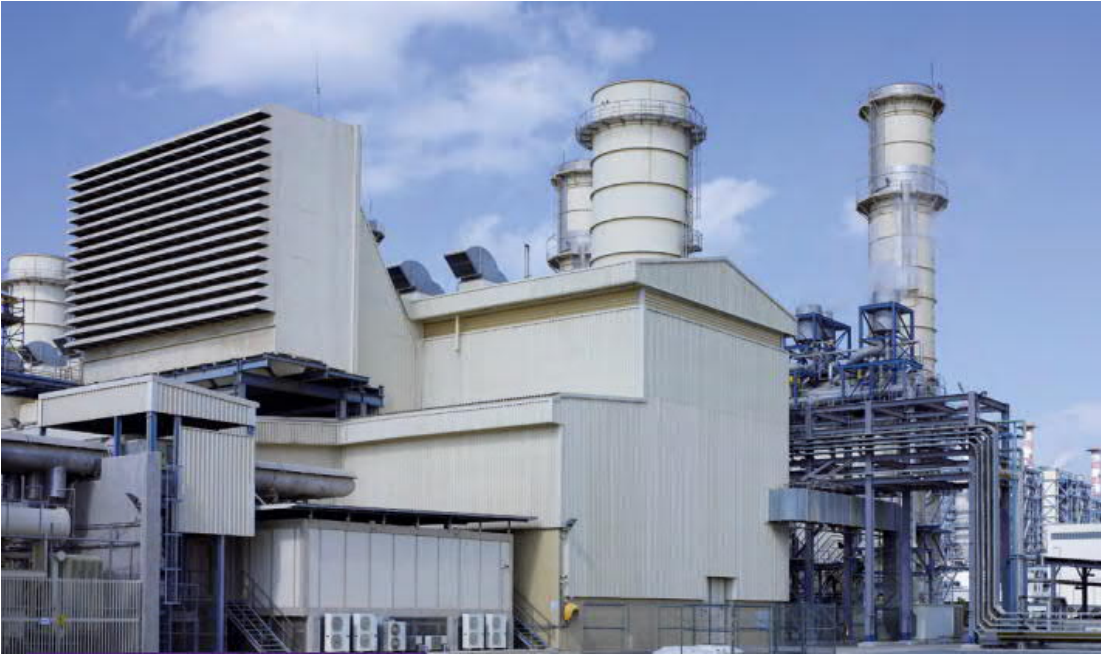
Figure 1.2: Image of a Typical OCGT Development
