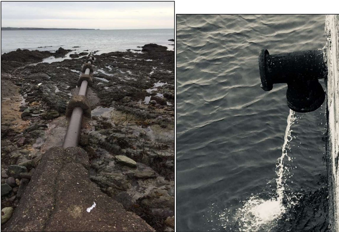
Figure 1-3: Views of the current waste water outfalls near the Cow slipway (left) and Ballycotton pier (right).
