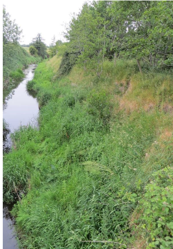
Photo 2: Erosion along the bank at the bridge.
