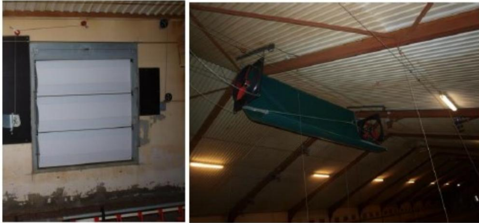
Example of slats (Louvre system) in the side wall and air collection in the ridge.
