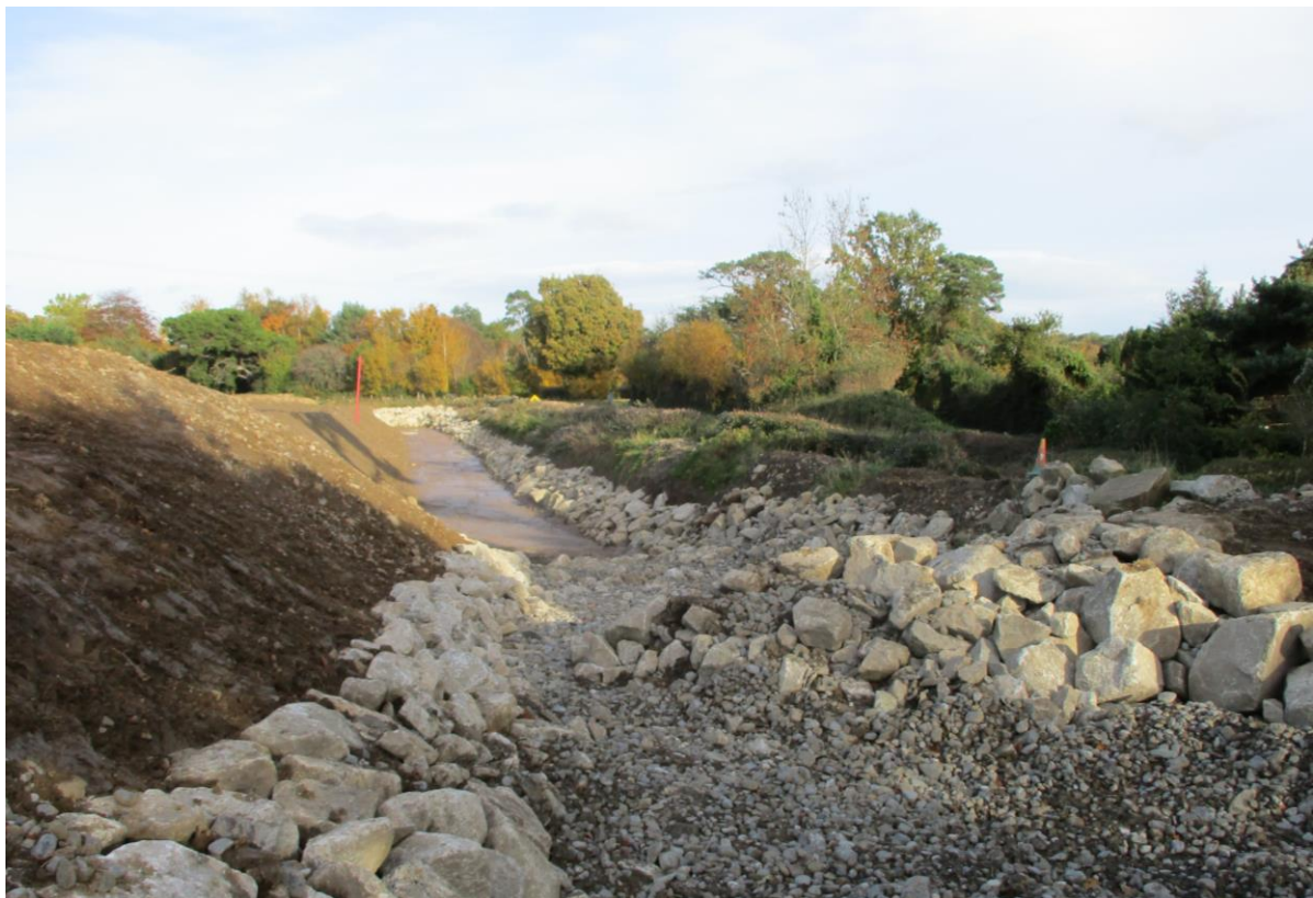
Plate 6 – View from Existing Channel to Holding Pond Upstream of Manhole / Pipe Drain
