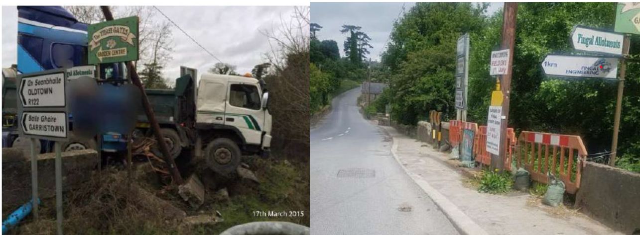
Figure 18 - On 17/03/2015 two trucks enroute to a facility north of Naul Bridge collided with a portion of the bridge parapet wall. Regardless of countless requests to the county council it took three years for this to be repaired.
