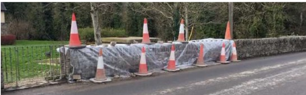
Figure 16 - Example of Traffic Hazard at Naul WWTP Site entrance. A truck collided with the bridge parapet wall on 29/01/2020. This is the parapet on the opposite side of the bridge from the WWTP site entrance.
