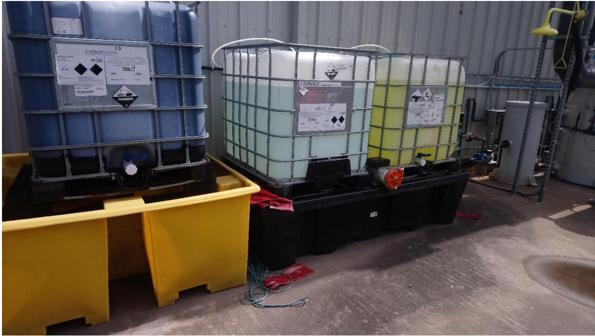
Photograph 5: Scrubber Treatment Chemicals Storage
