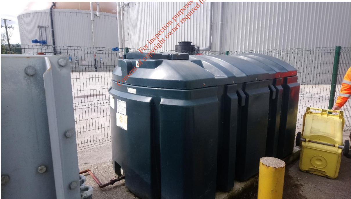
Photograph 2: Diesel Storage Tank Building 2
