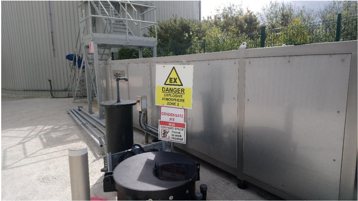
Photograph 13: 'Danger Zone' Condensate Pit
