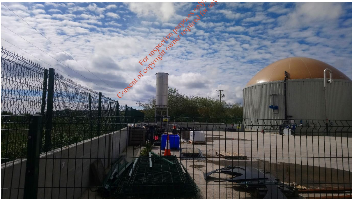
Photograph 10: Back-Up Gas Flare
