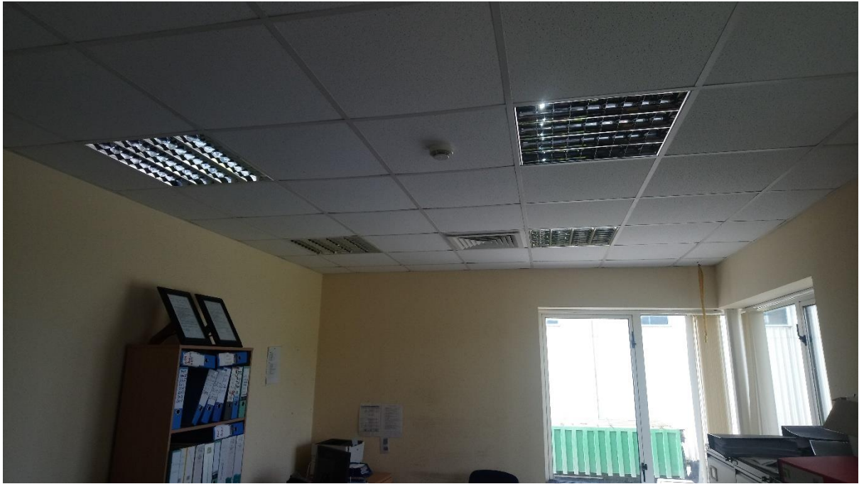
Photograph 1: Smoke Detectors in Office
