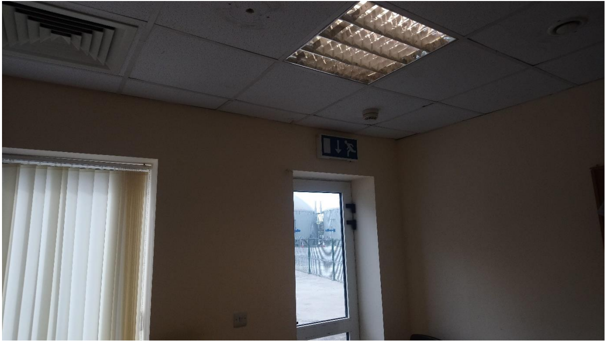
Photograph 5: Emergency Exit Signage-Office
