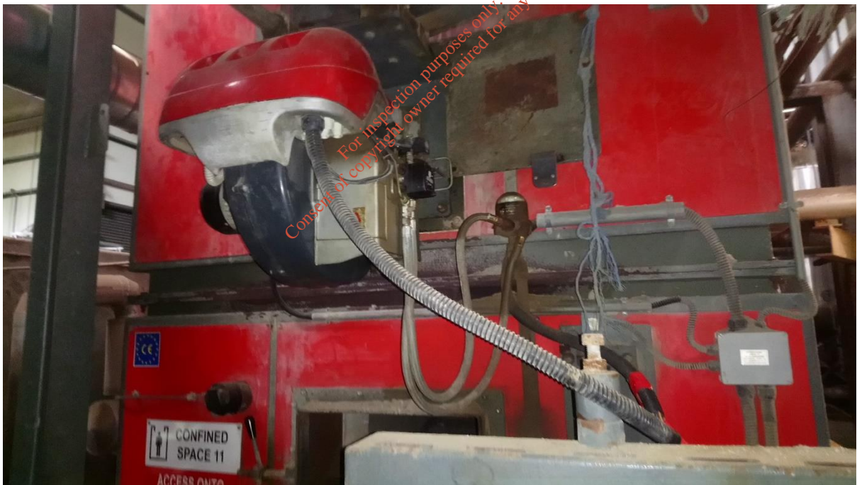
Photograph 28: Biomass Boiler Building 2
