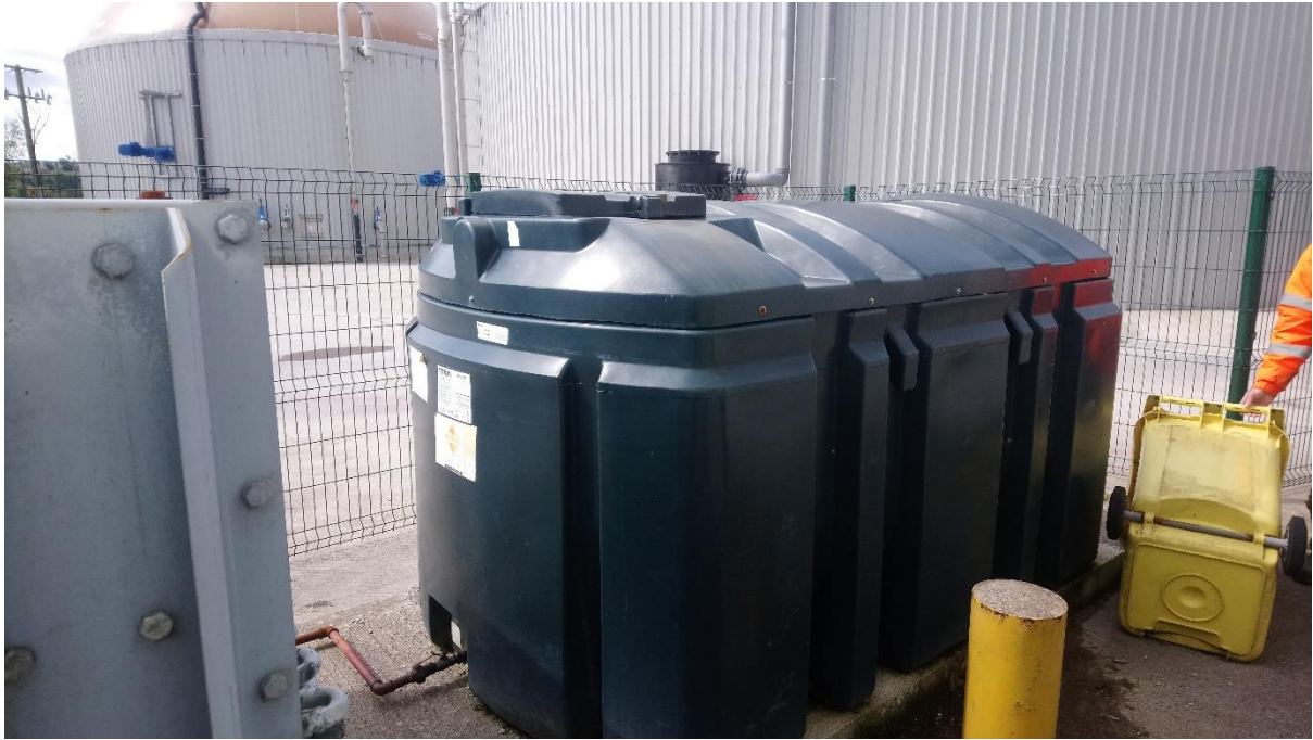
Photograph 15 : Above Ground Diesel Storage Tank & Spill Kit
