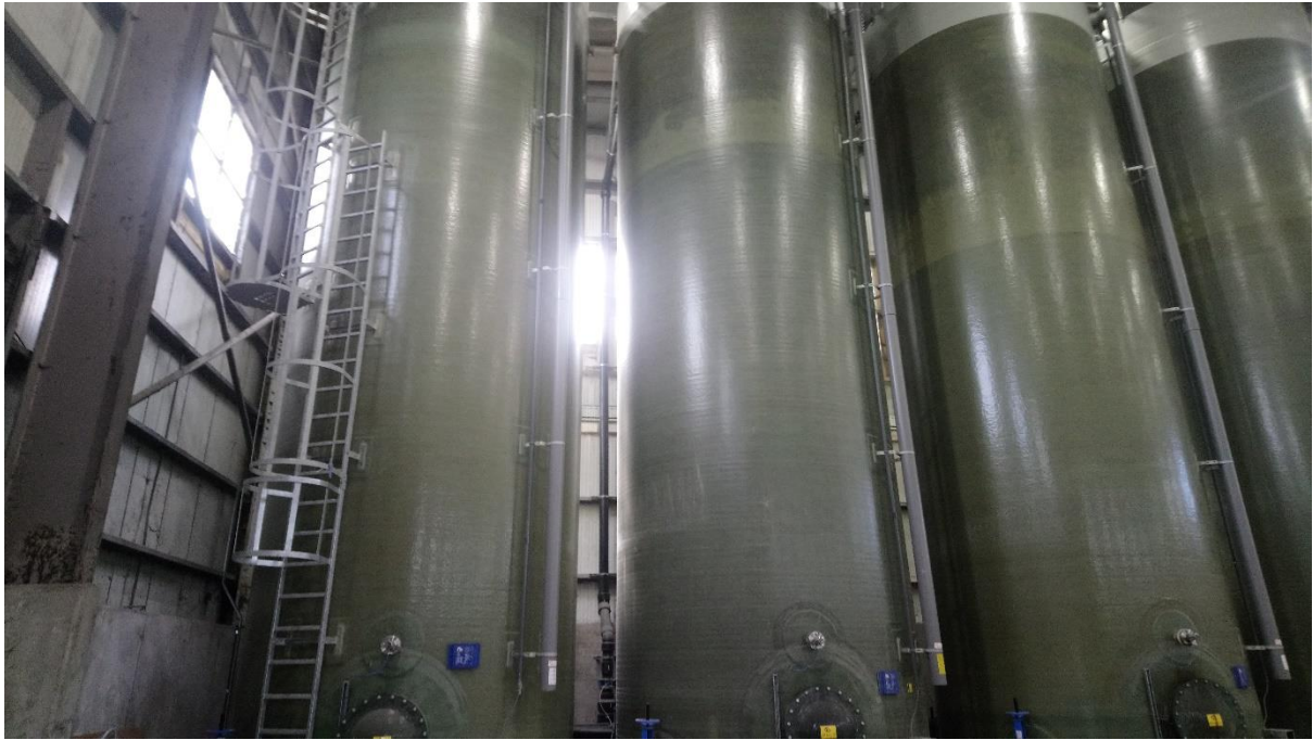
Photograph 21 : Bulk Liquid Waste Storage Tanks Building 1
