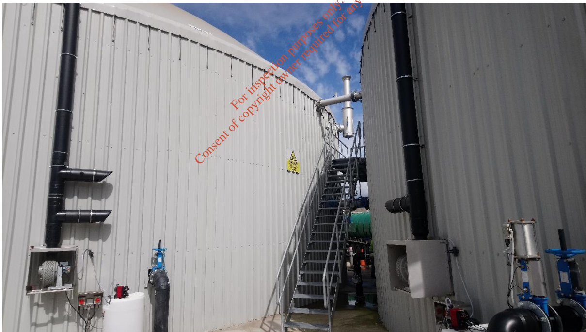
Photograph 14 : 'Danger Zone' Digester Pressure Release Valves
