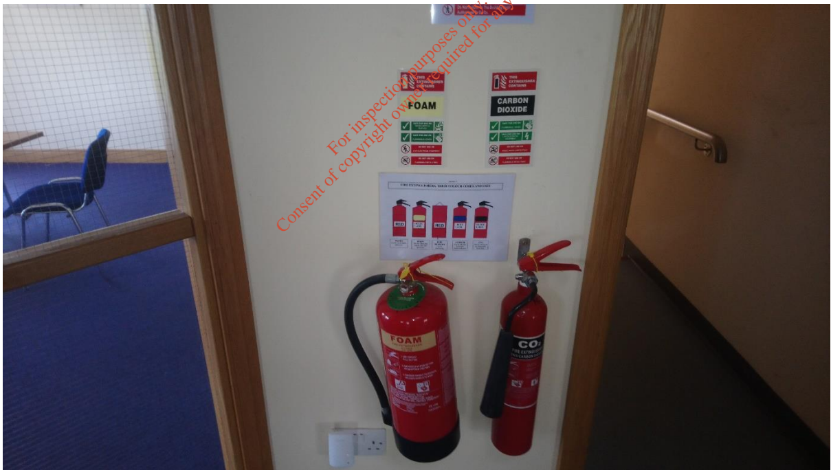
Photograph 2 : Fire Extinguishers in Office
