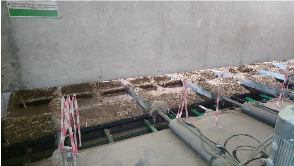
Photograph 29 : Residual Wood Chip in Biomass Boiler Feed Hopper Building 2
