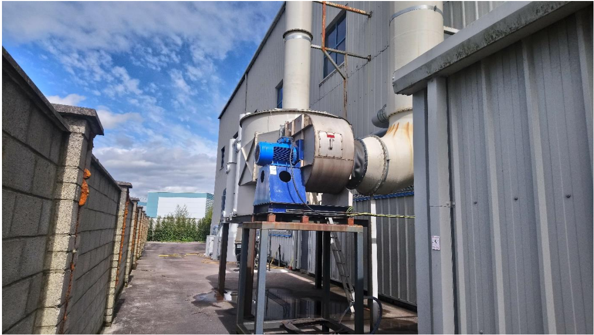
Photograph 19 : Odour Control Unit on Building 1
