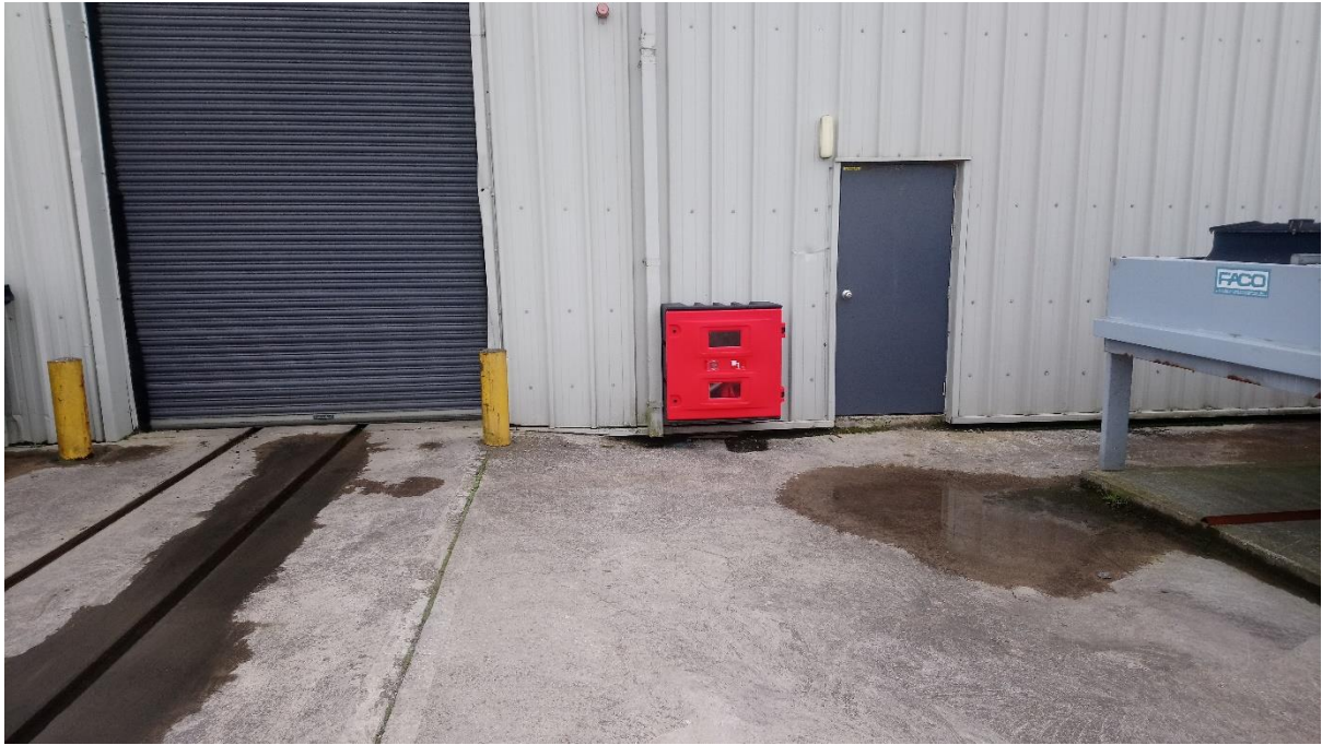
Photograph 17 : Hose Reel outside Building 2
