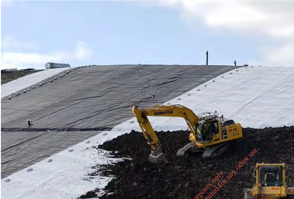
Figure 3-2: Landfill Capping: Placement of Subsoil atop Subsurface Drainage Layer (White) ,LLDPE Liner (Black) atop Landfill Gas Migration Layer (White -Far Left)
