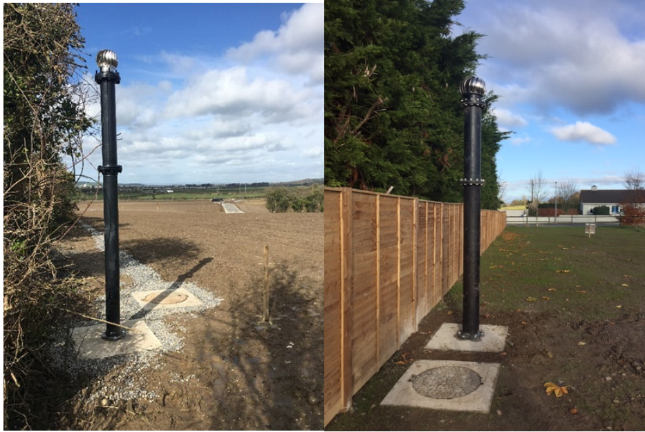
Figure 3-3: Typical Landfill Gas Ventilation Stack
