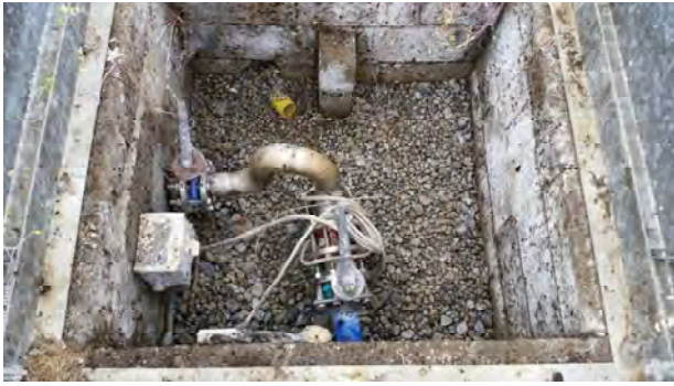
Photo 1. BH2 headworks in pump chamber
