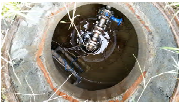
Photo 3. BH4 headworks in pump chamber. Note water ingress to borehole
