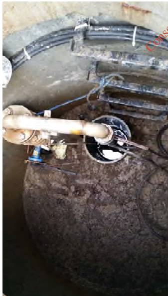
Photo 5. BH6 headworks in pump chamber.
