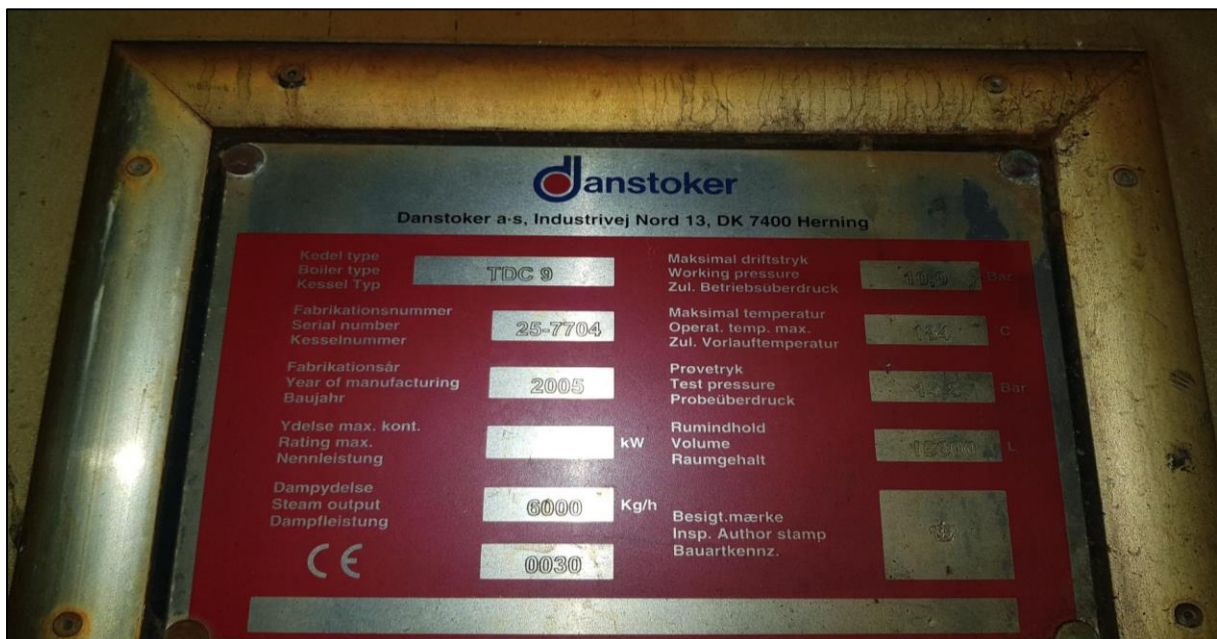
Figure 2-1: Duty boiler label
