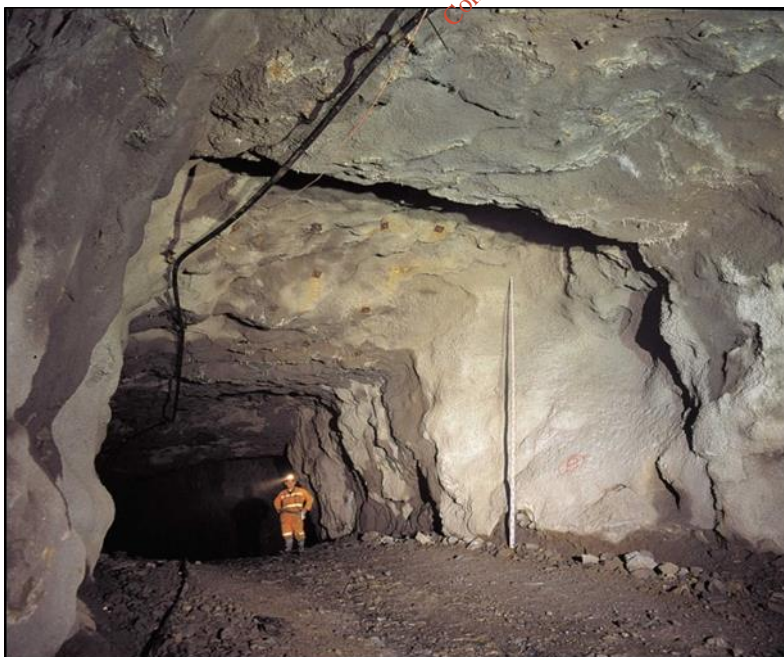
Figure 37: Shotcreted Fissure underground at Galmoy
