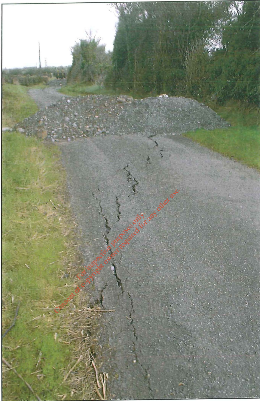
Photo 3. Tension cracks at the north end of the closed section of the road.
