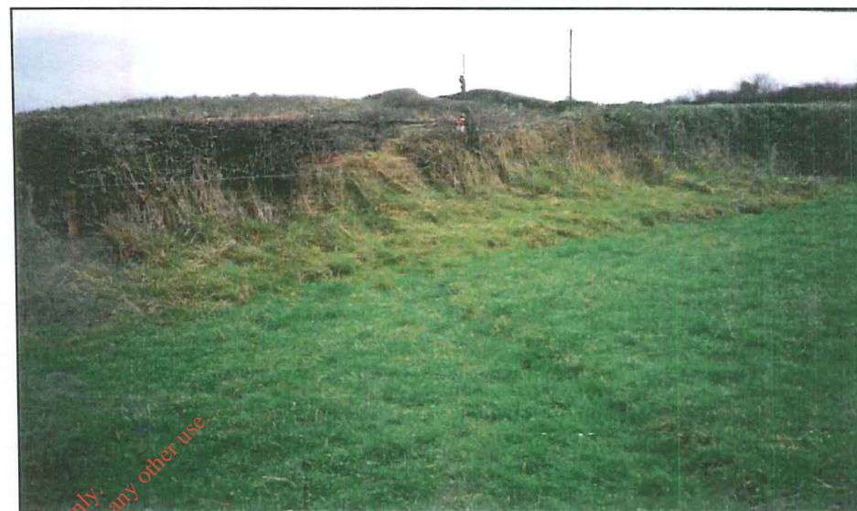
Photo 7. The north-westward extension of the open crack in the adjacent field.
