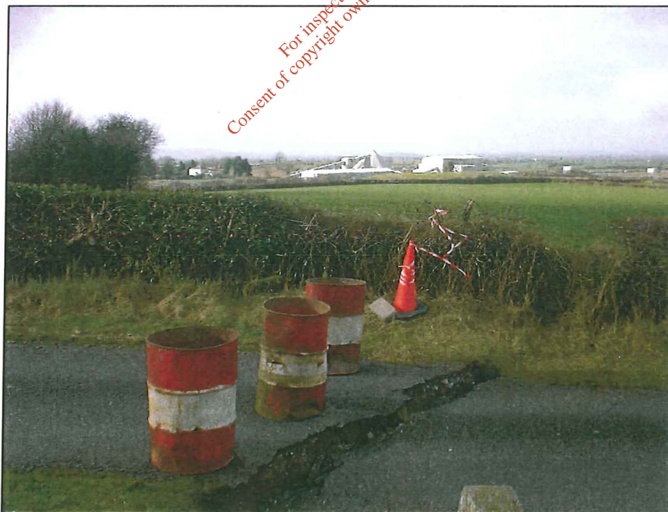
Photo 2. Vertical displacement on the open crack at the top of the hill, with the Galmoy facility in the background.
