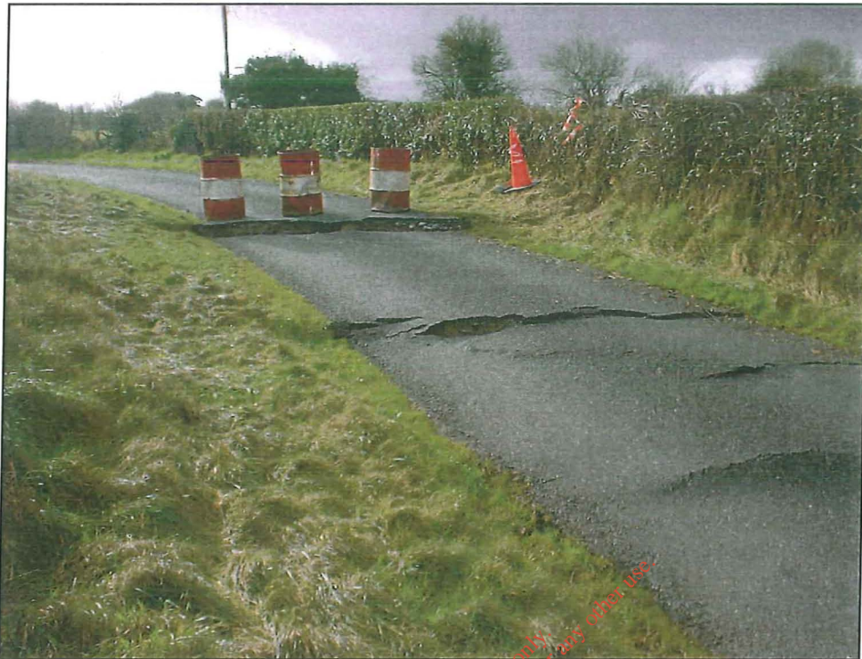
Photo 1. Damage to Whiteswall Road showing the open crack (top), the tension cracks (middle) and the pressure ridge (foreground).
