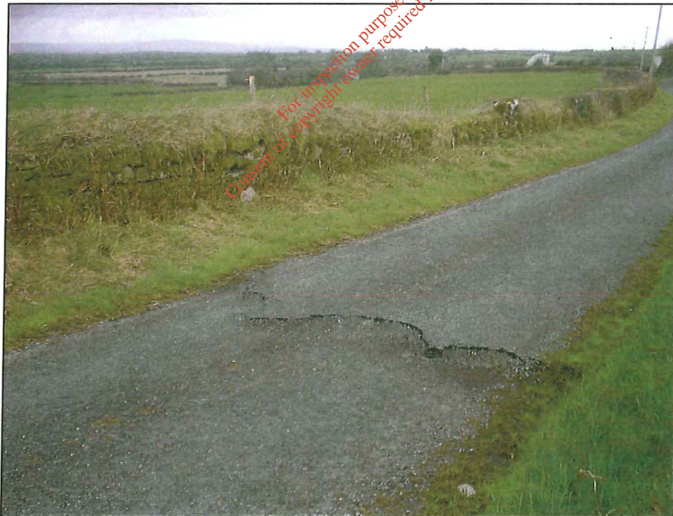
Photo 10. The cracked axis of the central pressure ridge, looking north, in early March.
