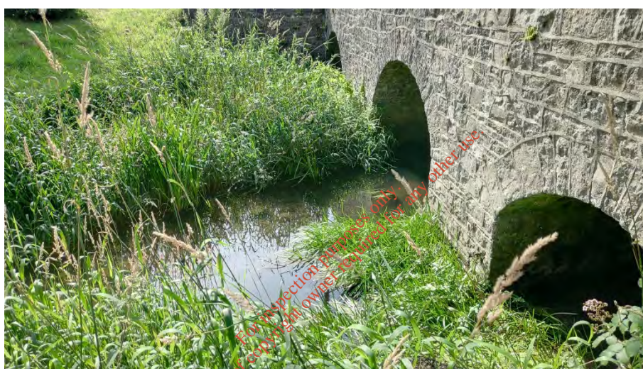
Plate 3.3 Representative image of site 3 on the River Nanny downstream of the R153 road bridge approx. 3.6km downstream of the Knockharley Landfill site boundary on 2 nd August 2019.
