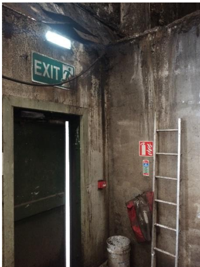
Plate 4: Fire Emergency Door at Acorn
