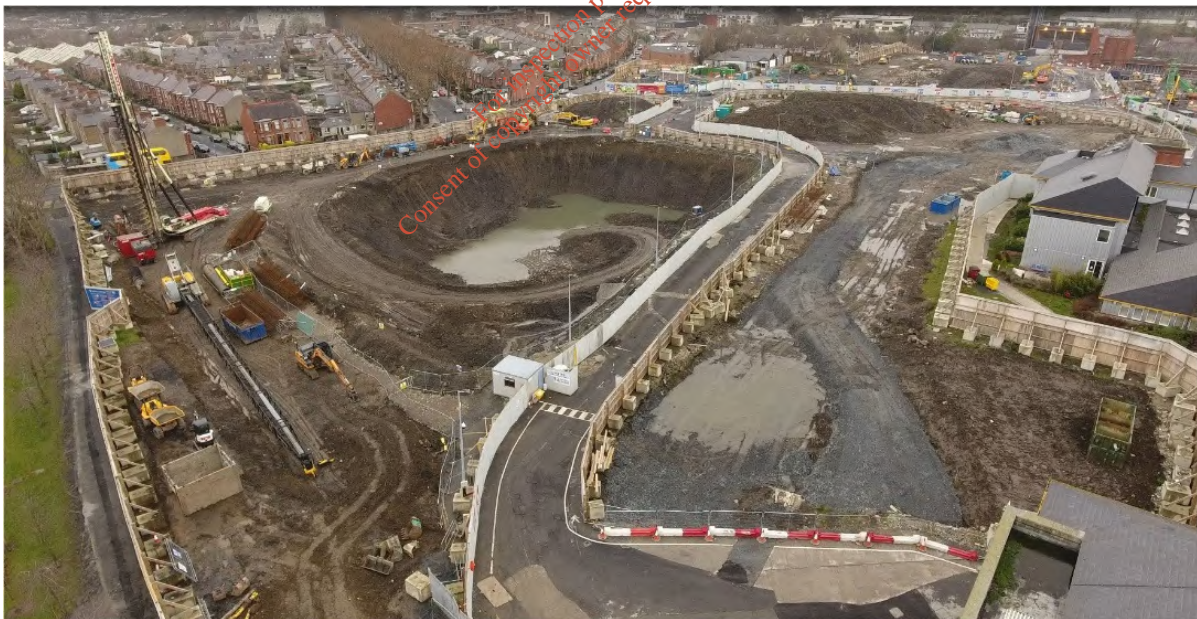
Plate 2: 4K Aerial photograph of NCH/St. James Hospital construction site facing NW on 2 nd January, 2018
