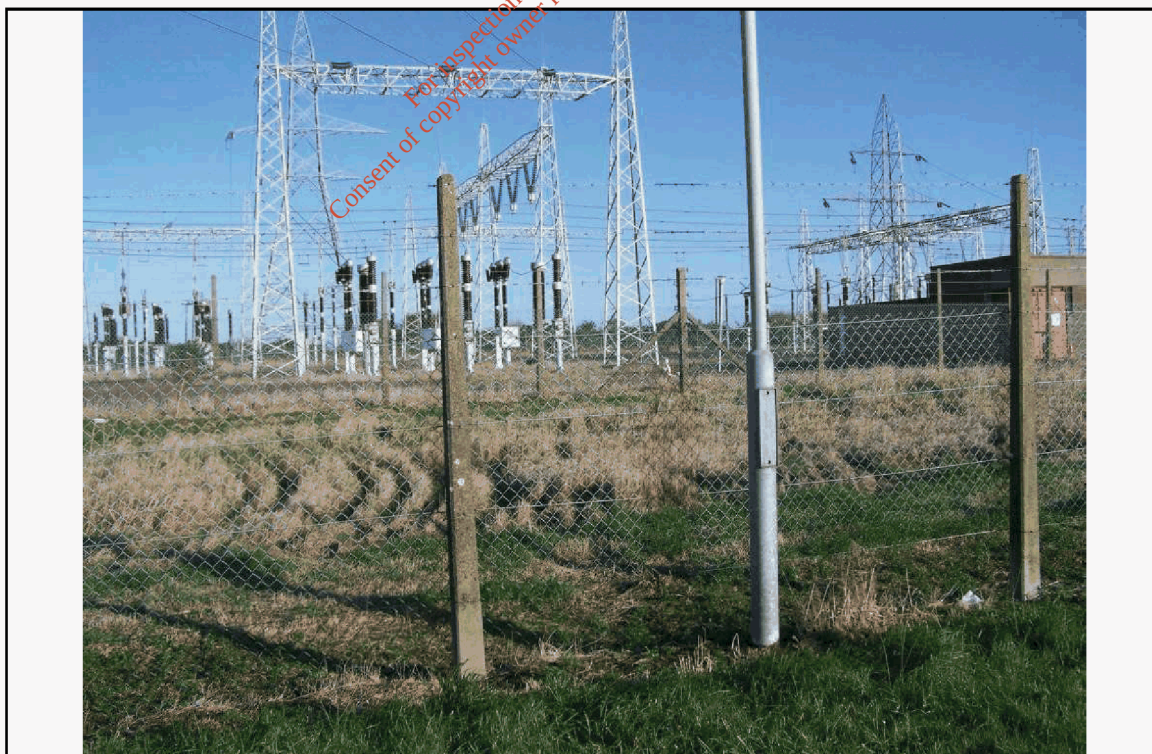
Location No: 22 View north 220kV switching yard.
