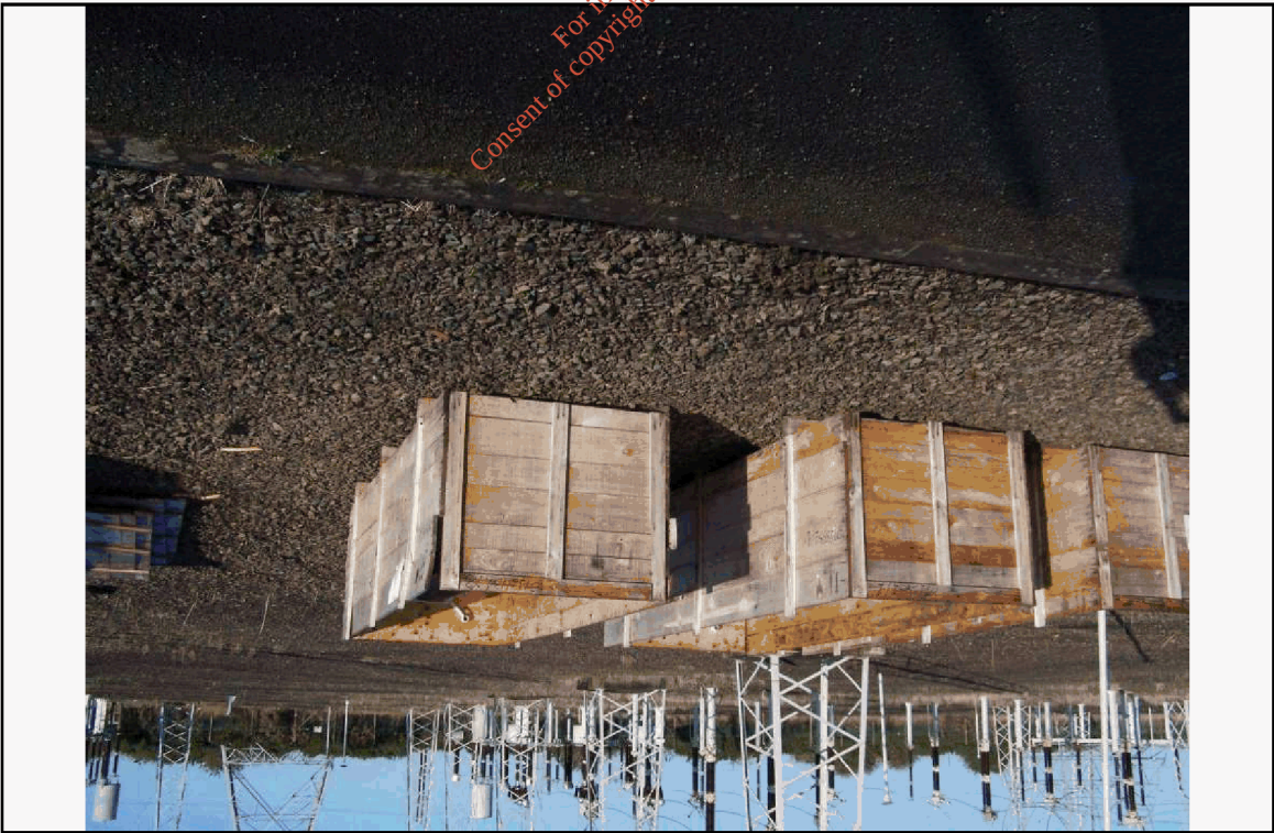
Location No: 10 View north 220 kV switching yard.
