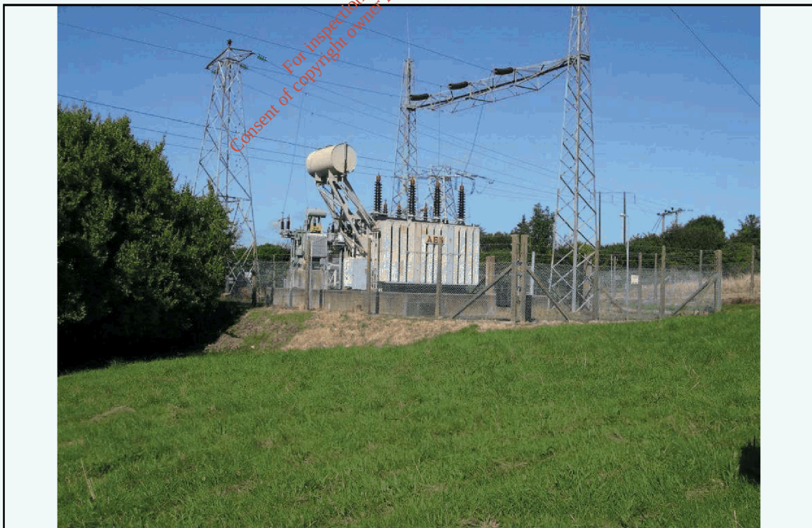
Location No: 24 View northwest 110 kV switching yard.
