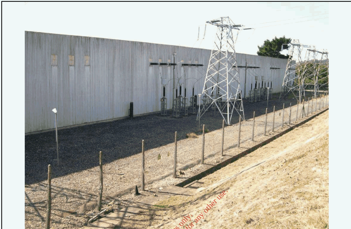
Location No: 23 View southwest 110 kV switching yard.
