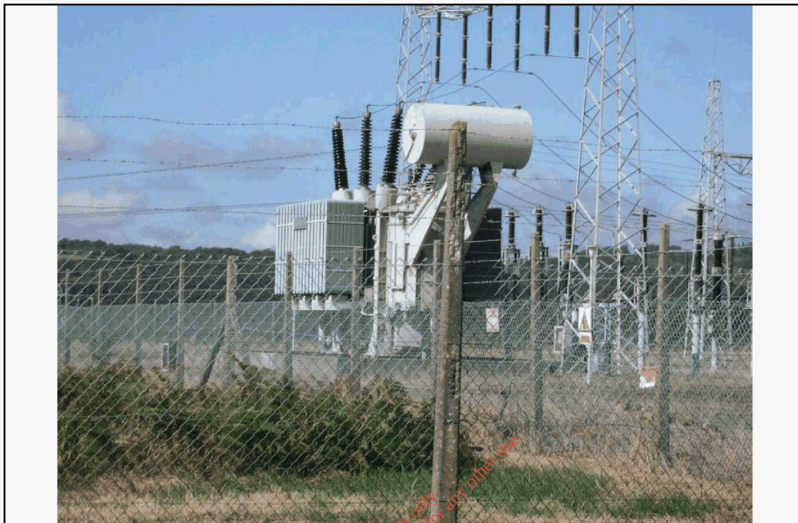
Location No: 22 View northwest 220kV switching yard.
