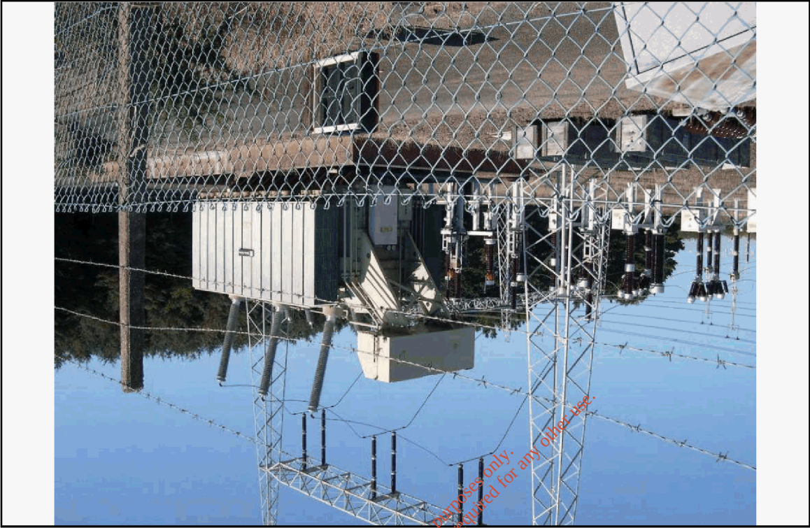
Location No: 11 View northeast 220 kV switching yard.
