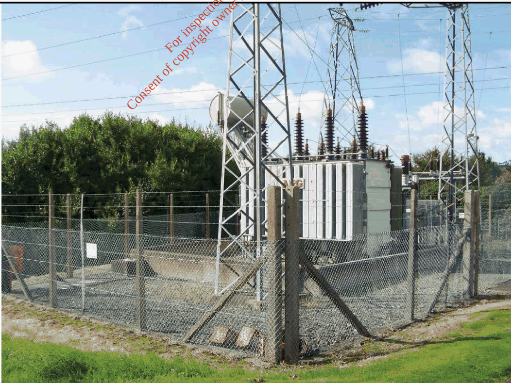
Location No: 13 View southwest 110 kV switching yard.
