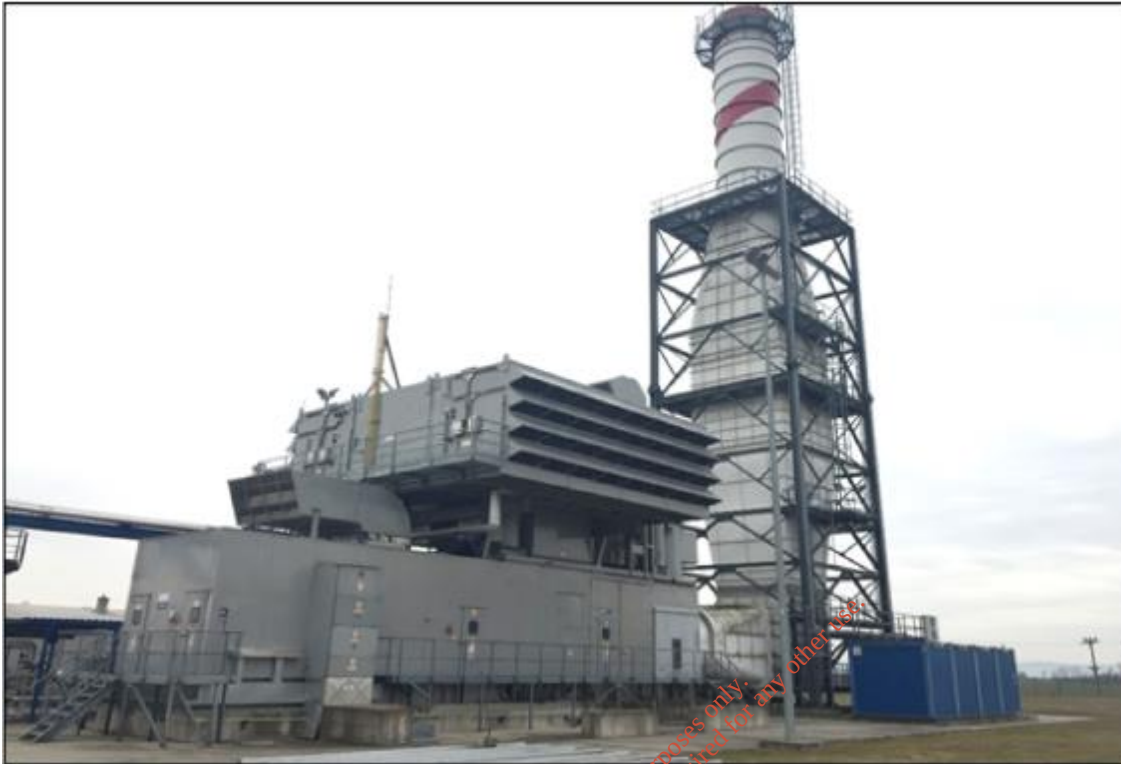
Figure 5.1: Typical FlexGen Unit
