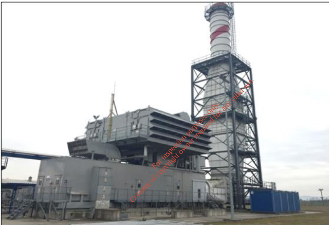
Figure 4.1: Typical FlexGen Unit
