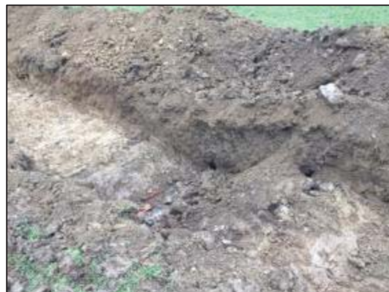
Plate 2: Detail of the land drain pipe revealed in trenches 1 and 2, from the south-west.
