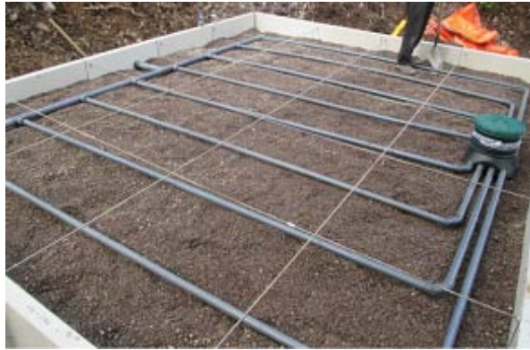
Fig 4.0 Completed pipe network on a Sandcel before placement of final gravel layer
