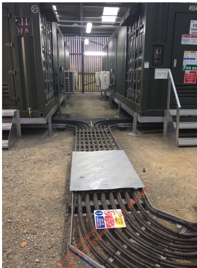
Figure 3-5 Example of Above Ground Cable Tray Installation
