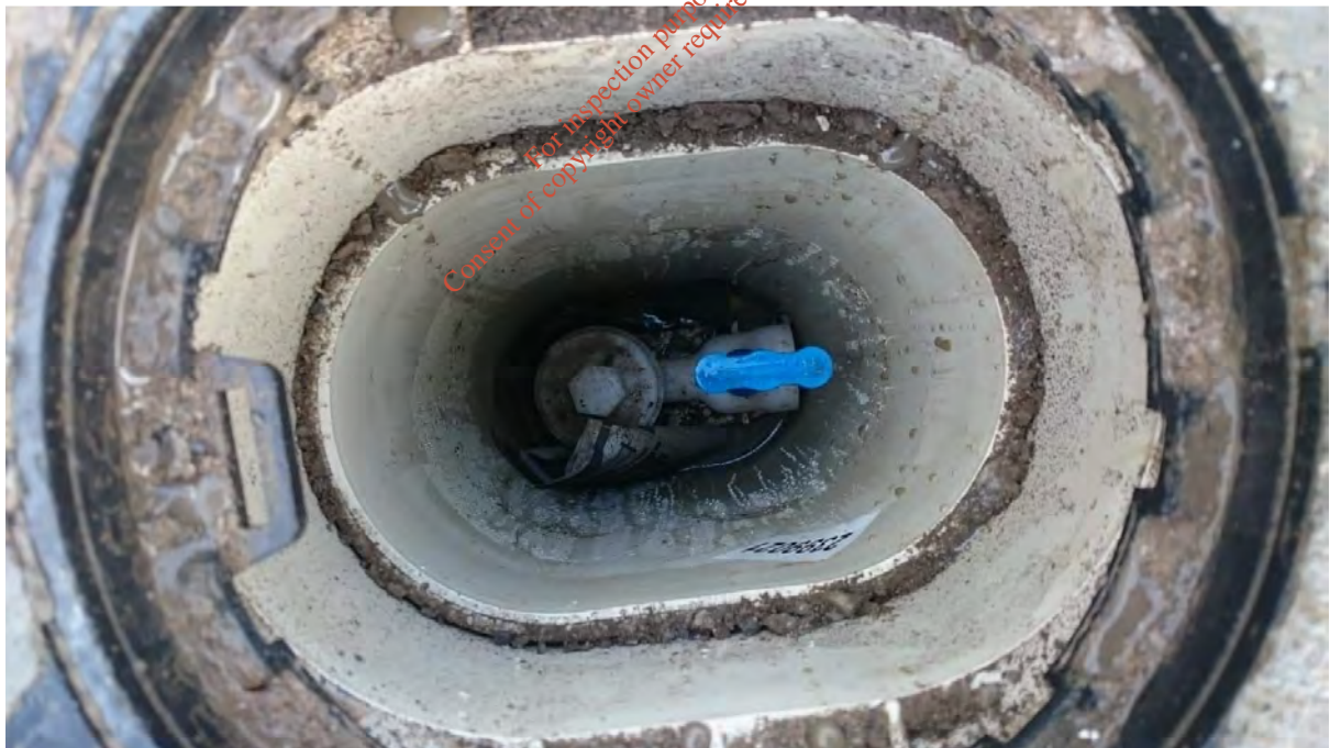
Plate 4: Closer view of water main meter without frost protection plug
