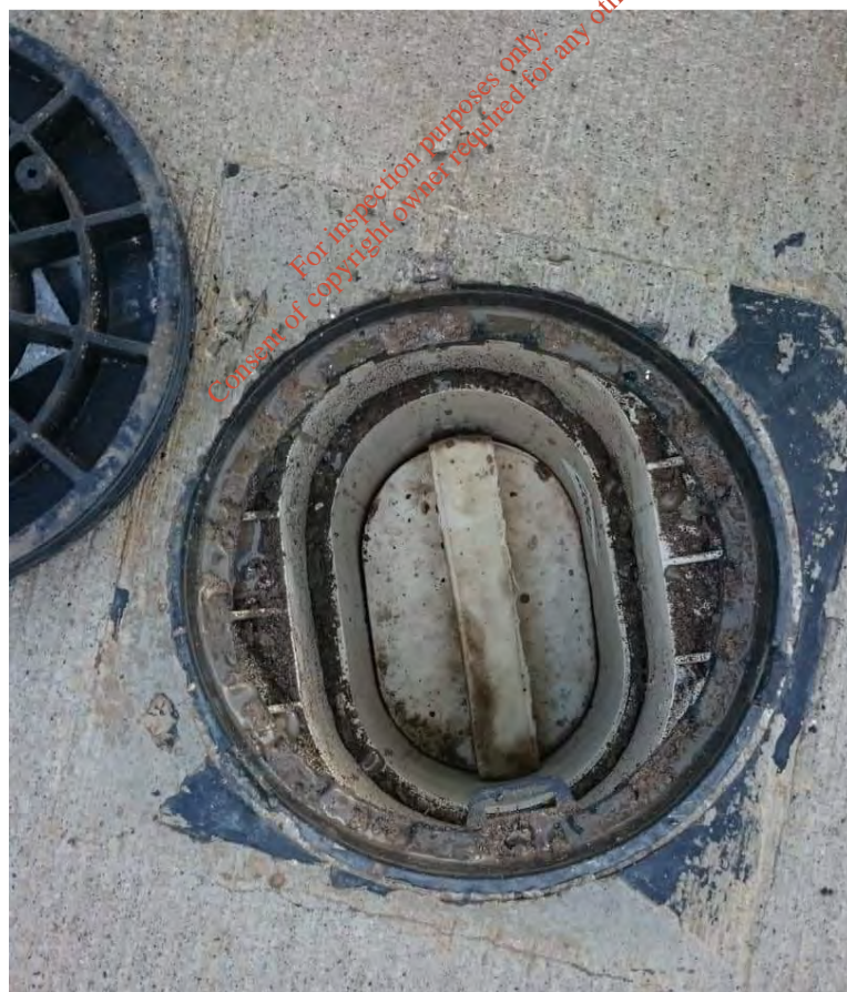
Plate 2: Water main meter box with black HDPE circular cap removed
