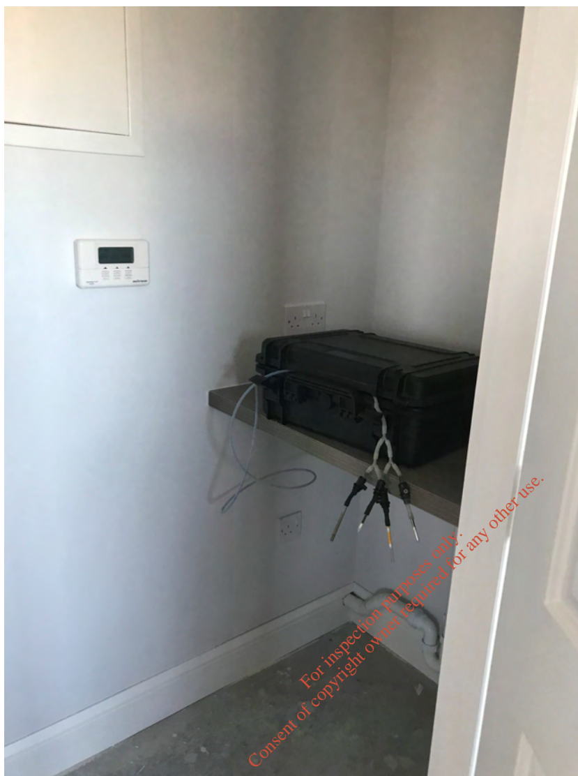
Figure 7.2. Location of monitoring in Hse 25, Utility
