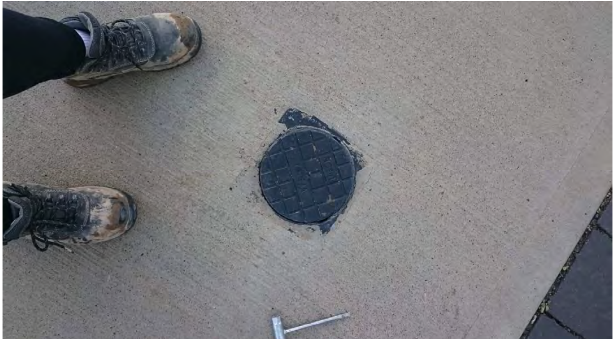
Plate 1: Water main meter box viewed from above
