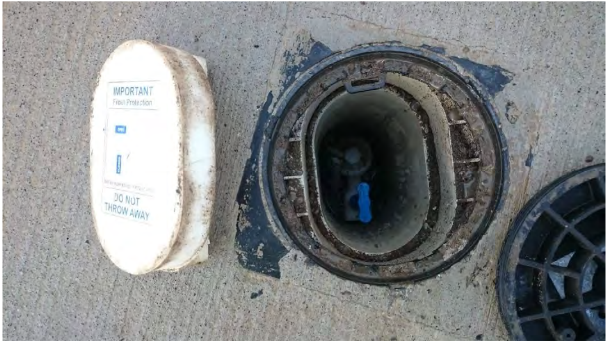
Plate 3: Water main meter box with black HDPE circular cap removed and frost protection plug removed (see to left)
