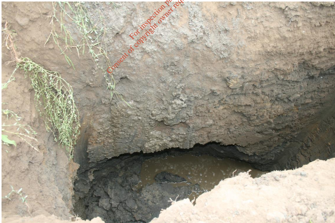
Plate A7.18 Photograph of soil profile from TP48 showing subsidence and groundwater ingress
