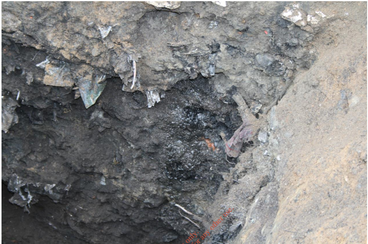
Plate A7.5 Photograph of hydrocarbon staining on trialpit wall (TP7)
