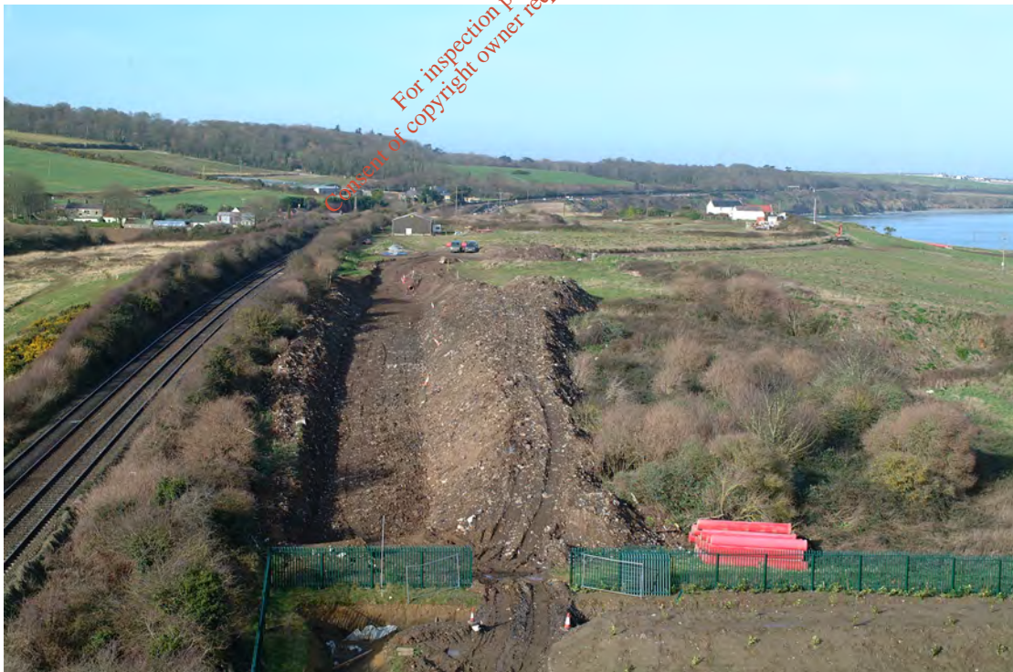
Plate A2.2 Photograph of excavation of soils for Rising Main taken in 2005 from western boundary facing west with Dublin-Belfast railway line to the south and historical landfill located to the north
