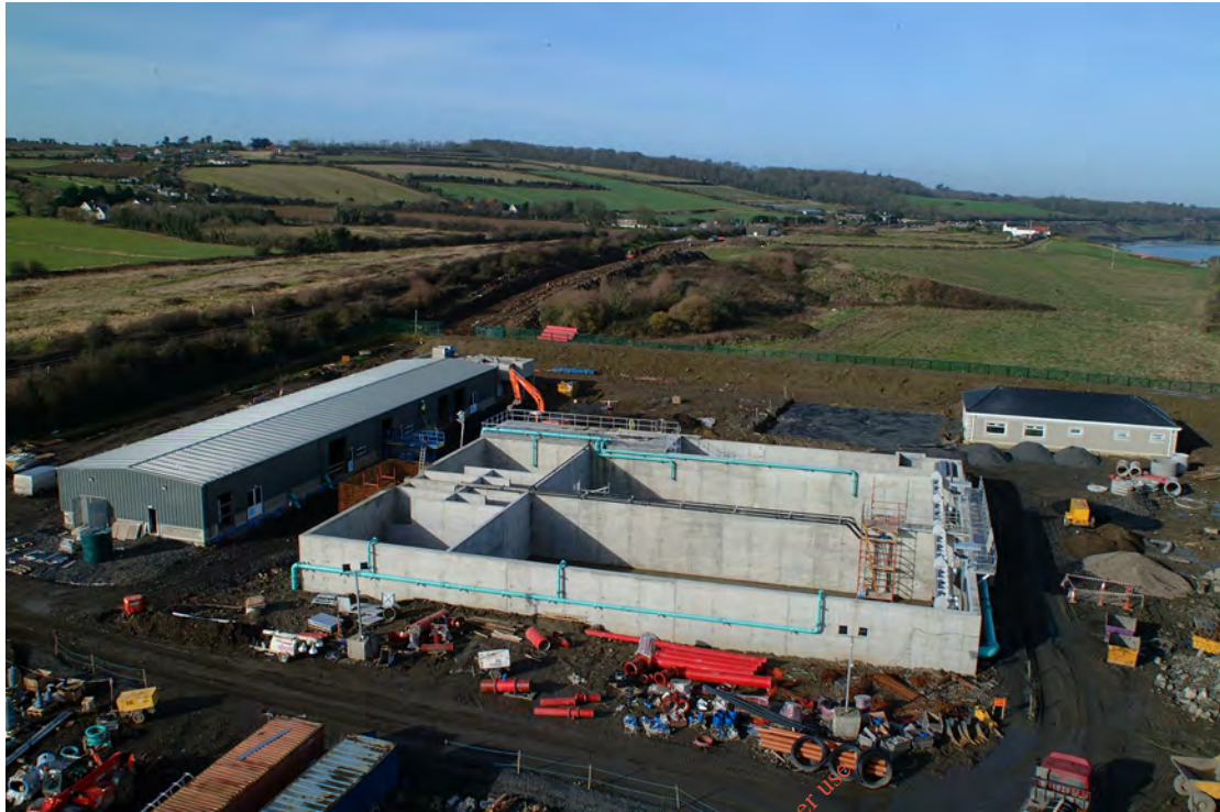
Plate A2.1 Photograph of Construction of WWTP and Rising Main taken in 2005 from western boundary facing west with Dublin-Belfast railway line to the south and historical landfill located to the west
