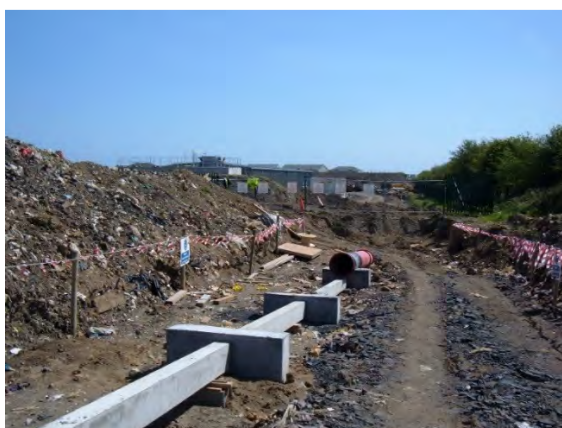
Plate 6. Photograph taken during rising main construction through waste body on 28/4/2006 (facing SE from subject site towards WWTP under construction)
