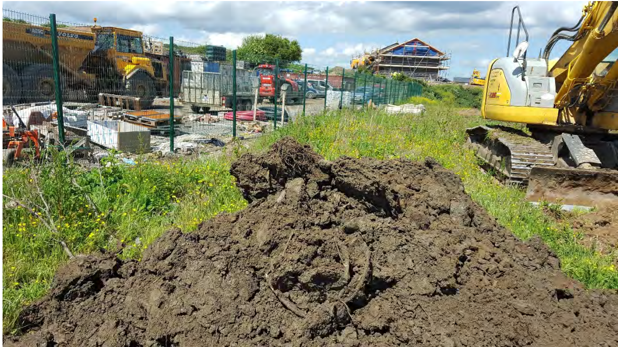
Plate 25. Soil stockpile of trialpit, TP25 excavated to the north of the builders compound
