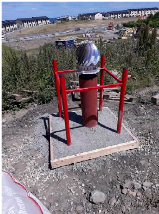
Plate 10. Gas venting well GV4 facing northwards towards builder's compound
