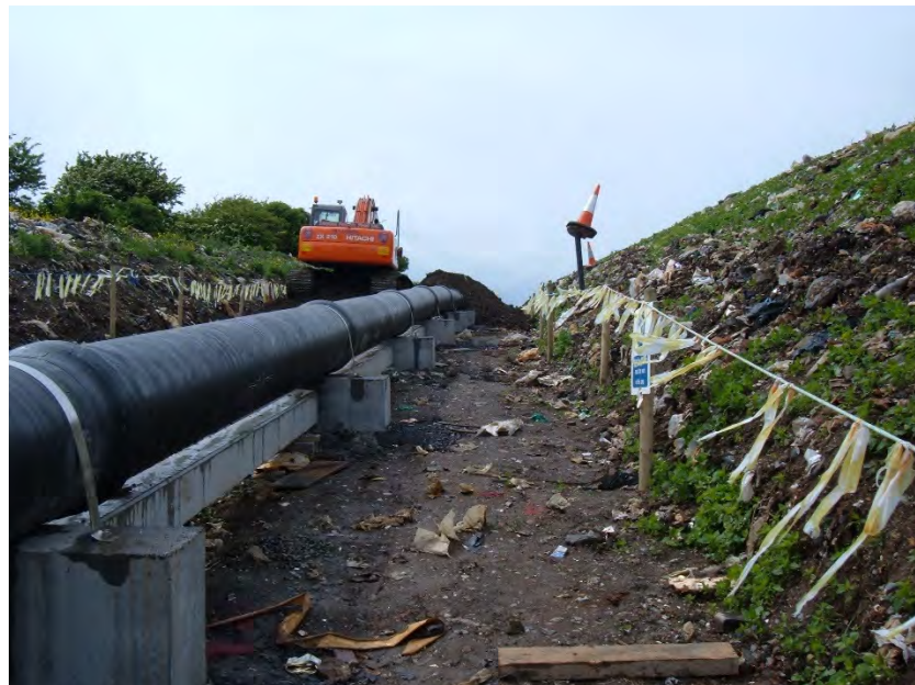
Plate 7. Photograph taken during rising main construction through waste body on 23/5/2006 (facing NW from eastern boundary of site with railway line to the left)
