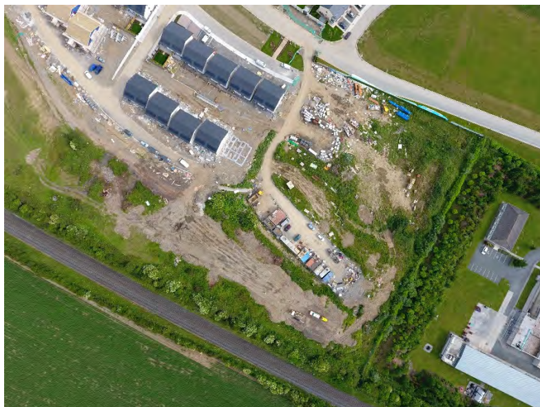
Plate 11. Historic landfill with newly built residences located to the north and northeast (note that the construction of Residences No. 25 and 26 required a piled foundation prior to subsequent completion)
