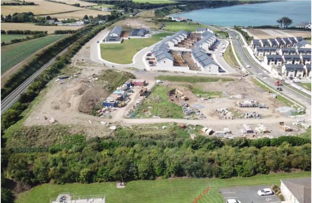
Figure 2.3 Barnageeragh Landfill Site (looking west) during the construction of the Hamilton Hill housing development
