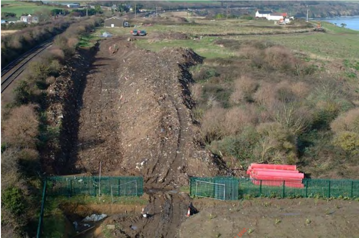
Figure 2.1 Barnageeragh Landfill During Construction of Wastewater Rising Main (view to the west, 2006).
