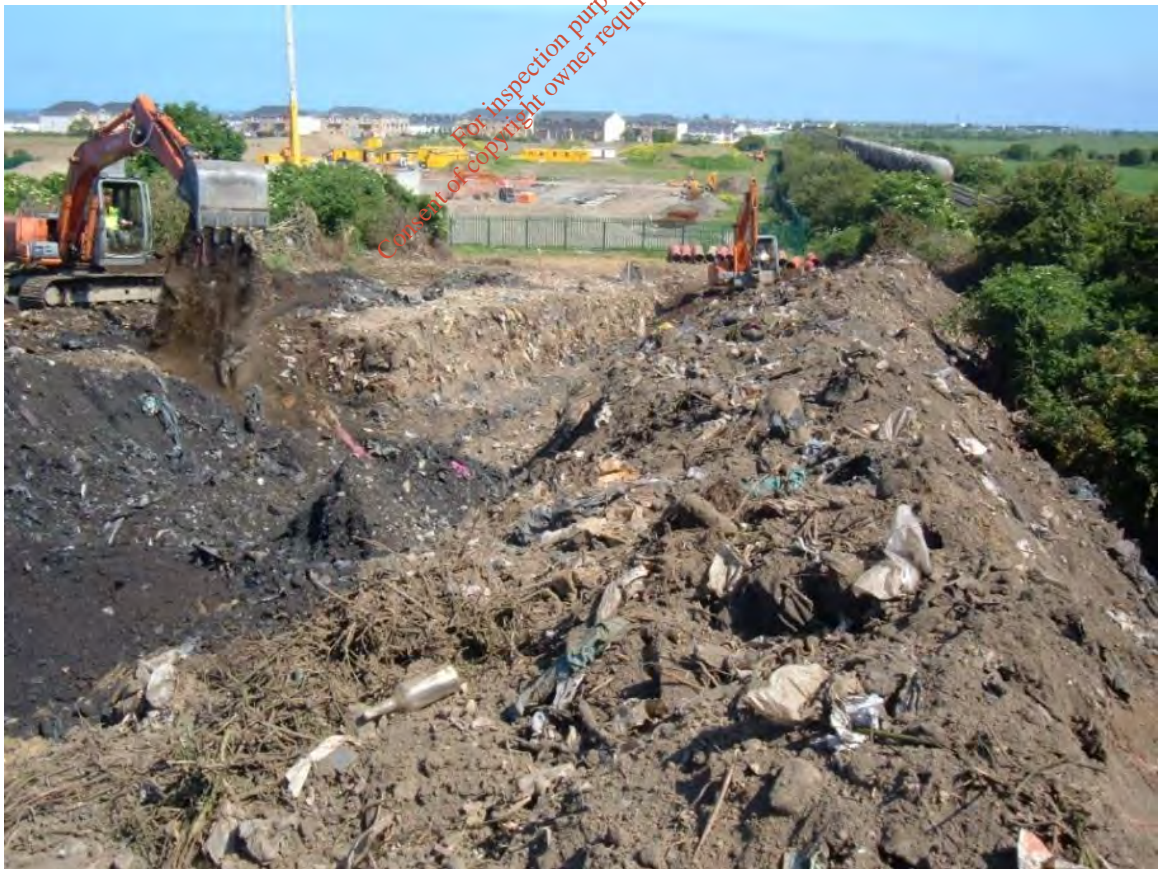
Figure 2.2 Barnageeragh Landfill During Construction of Wastewater Rising Main (view to the east, 2005).
