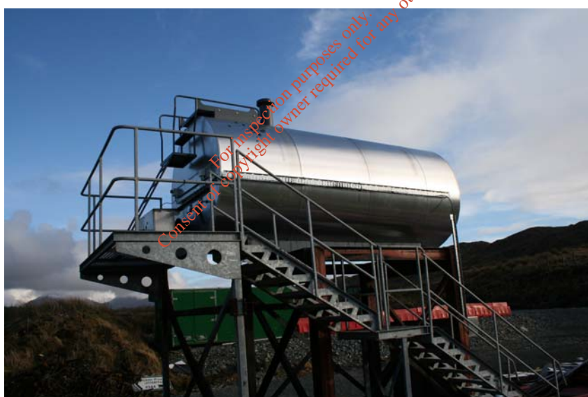
Plate 3. View of 10,000l aboveground storage tank used for the storage of road bitumen
