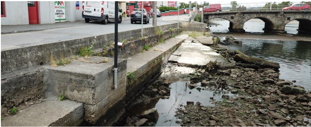
Figure 13.13: Poor condition and presentation of quay wall downstream of Arklow Bridge
