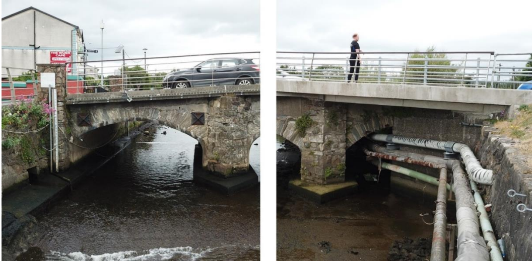
Figure 13.8: Downstream view of the first (southern) and nineteenth (northern) arch of the Arklow Bridge
