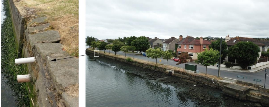
Figure 13.14: Section of quay wall where rubble stone remains visible and stone flags form top of wall
