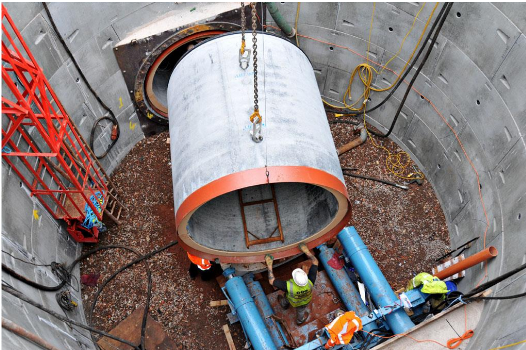
Figure 5.4: Typical setup of the jacking frame installing the pipeline in a tunnel shaft
