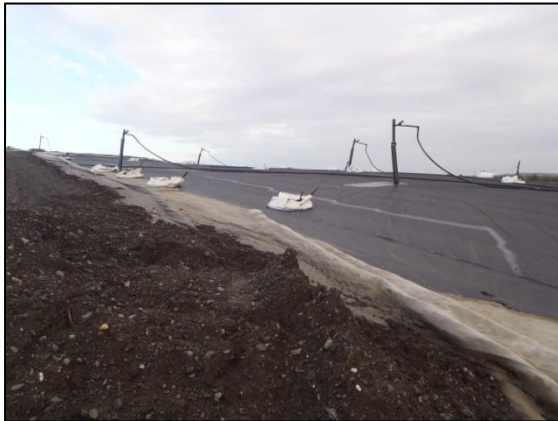
Plate 6 – Surface seal, cover soils and LFG collection infrastructure
