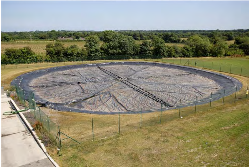
Plate 2-4: Covered Leachate Lagoon
