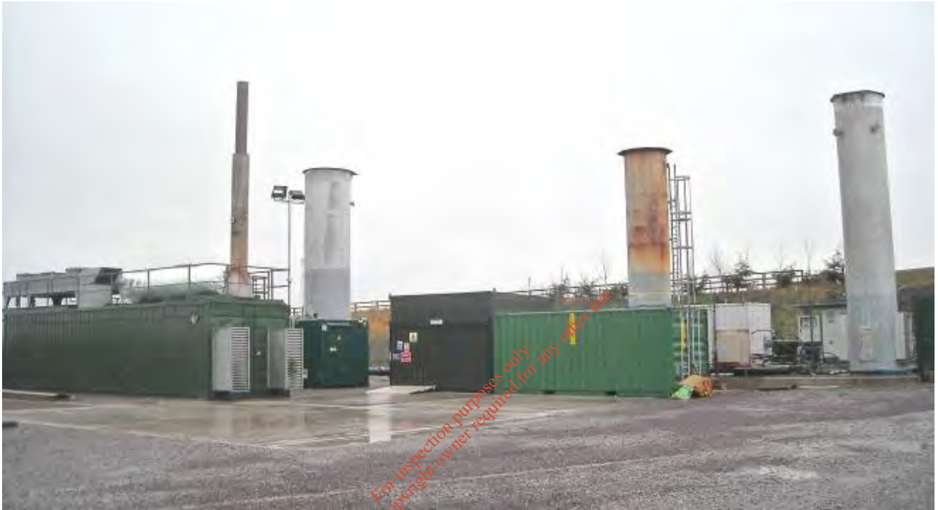
Plate 2-6: Landfill Gas Compound
