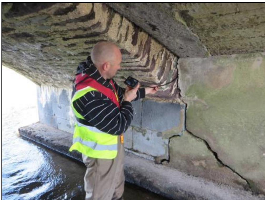
Plate 8 A borescope was used to investigate the crevices and cracks for any signs of roosting bats. No such evidence was found in any part of Finnow Bridge however.
