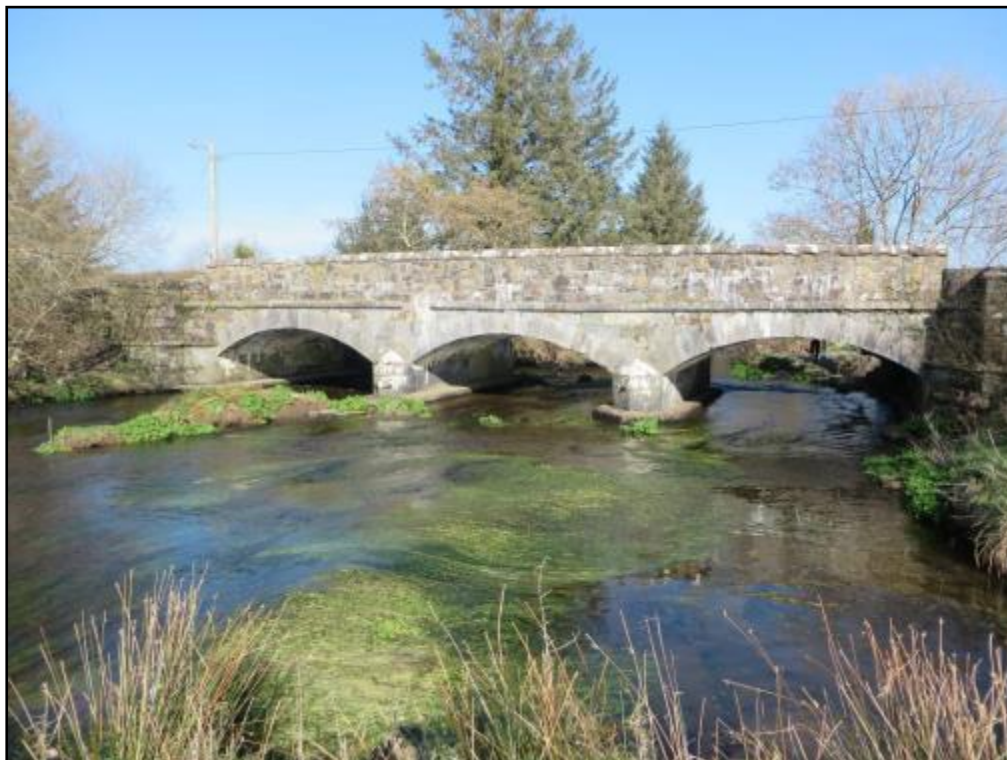
Plate 9 Upstream face of Finnow Bridge. This aspect of the bridge has no potential to be used by bats but the underside of the arches had crevices that could be used by bats for roosting.
