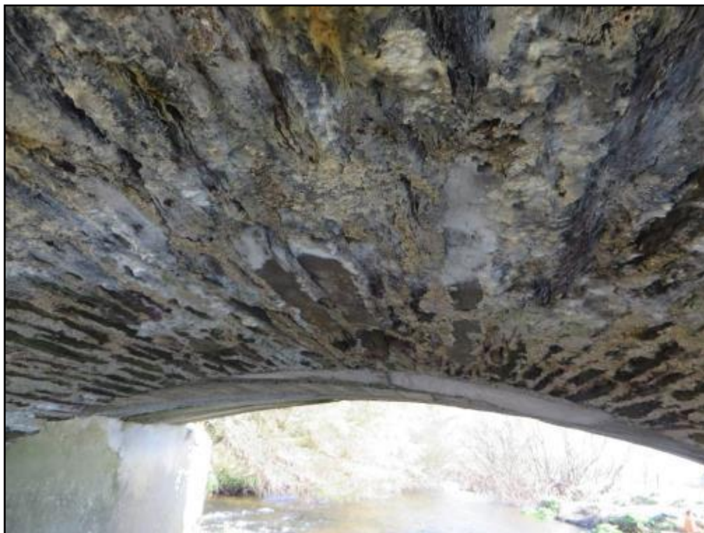
Plate 12 Stonework on the arches of the Finnow Bridge provided suboptimal roosting conditions for bats.
