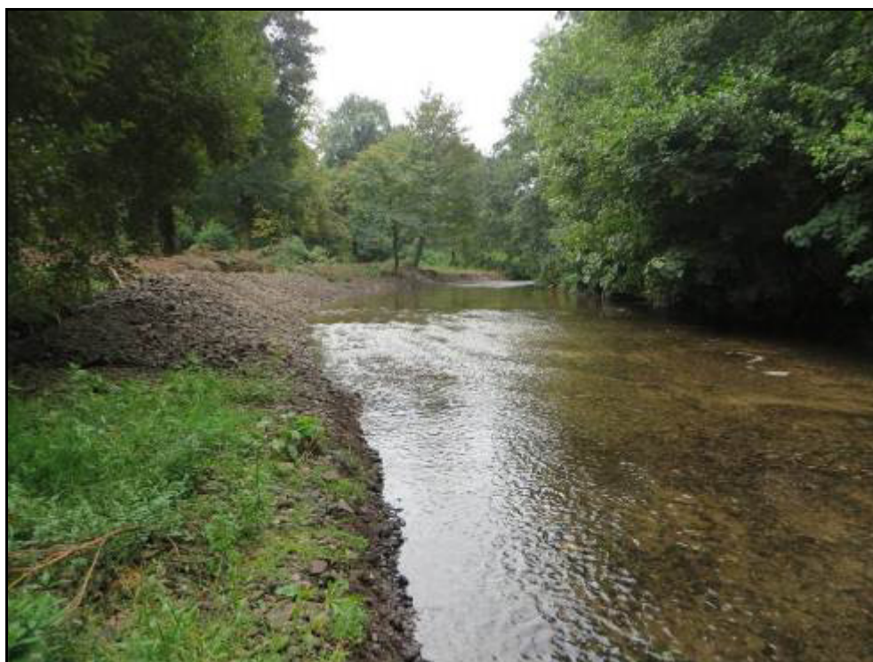
Plate 29 River Finnow approximately 200m upstream of Wallis's Bridge. This part of the river has been excavated and at the upper extent of the works area, the right bank has been re-graded using stones from the river.
