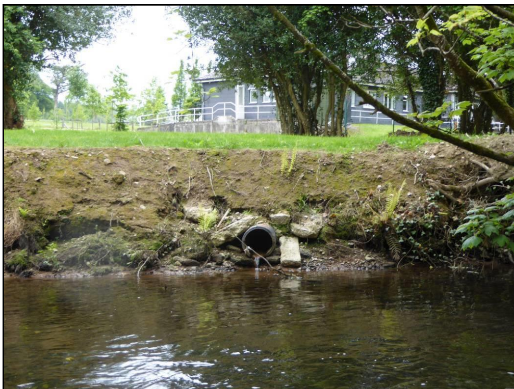
Plate 56 Outfall from the WwTP serving the new development at Drishane Castle.
