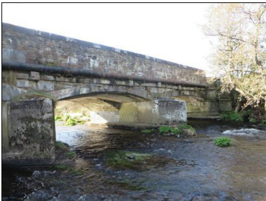
Plate 10 The downstream face of Finnow Bridge. Finnow Bridge has a number of crevices and cracks that were deemed suitable for resting bats.
