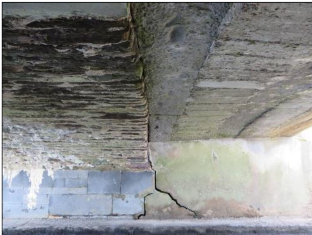
Plate 11 Crevices on the right arch of Finnow Bridge and a structural crack would provide potential habitat for roosting bats. However, no bats, bat droppings or other signs of bats were recorded during the survey.
