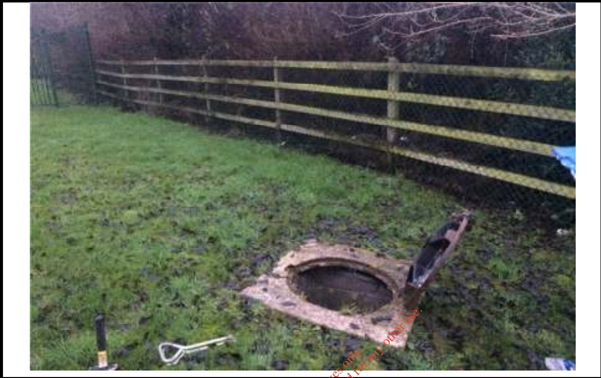
Photograph5 : Location No. 5 Surface Water Inspection Manhole.
