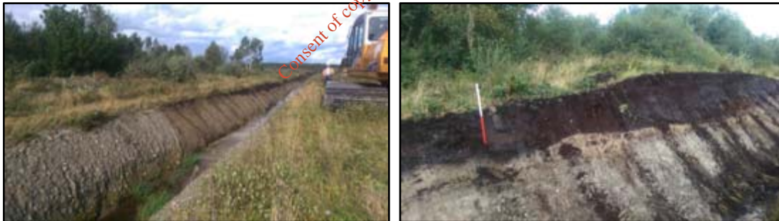
Plates 20 & 21: Details of drain 6 with silty sandy with frequent stones and peat.
