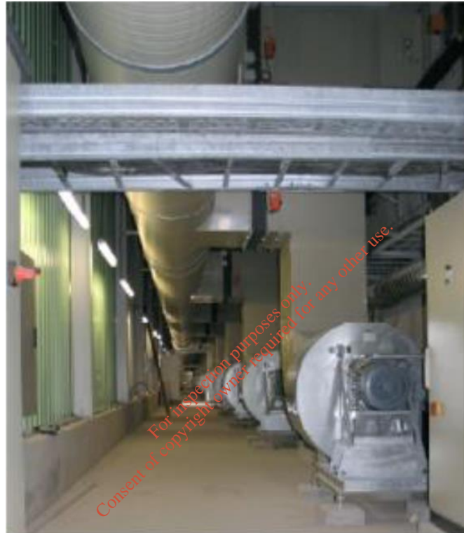
Figure 3.9: Typical Aeration Fan and Ductwork Installation
