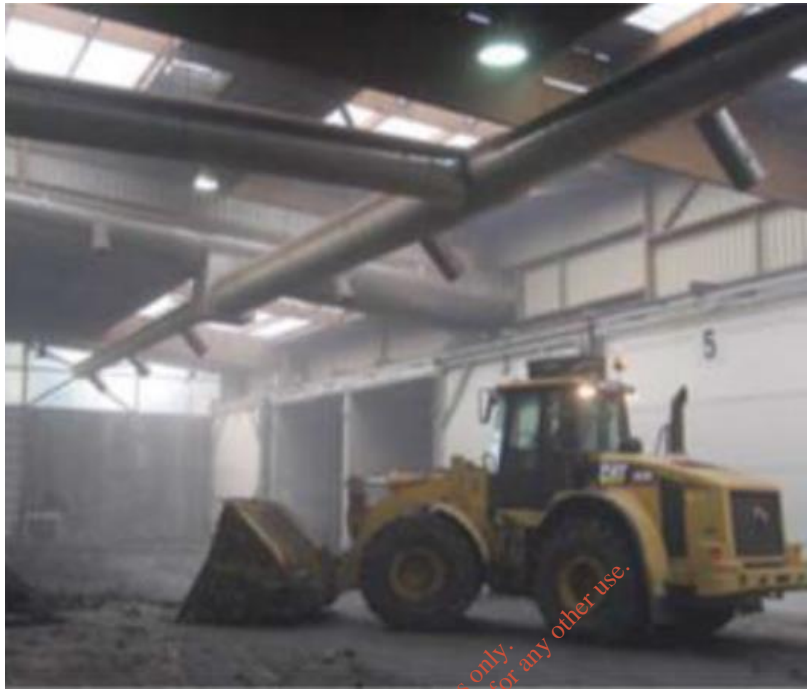
Figure 3.3: Loading of Dry AD Tunnels
