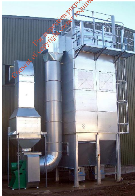
Figure 3.11: Typical Dust Filter System
