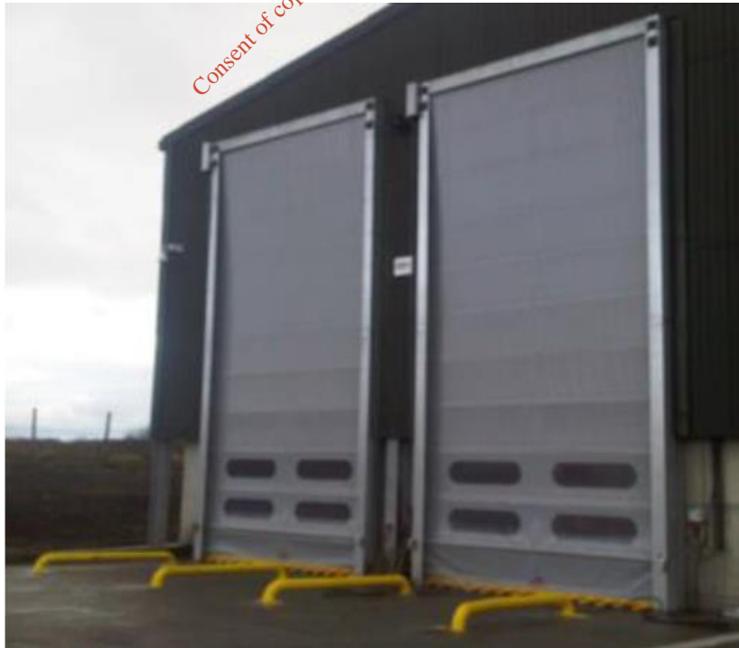
Figure 3.1: Typical Waste Receiving Doors
