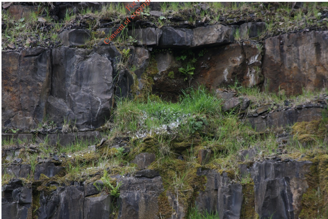
Figure 6. The first ledge identified on the southern boundary of the quarry. A number of fresh kills are evident on the front of the ledge.
