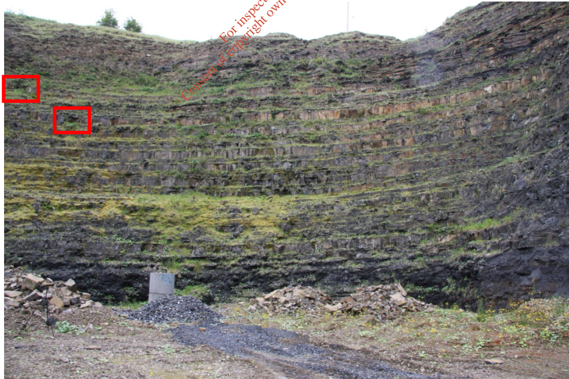
Figure 8. Cliff face showing the location of the two ledges identified on the southern boundary of the quarry. The ledge is located at the centre of the red box.
